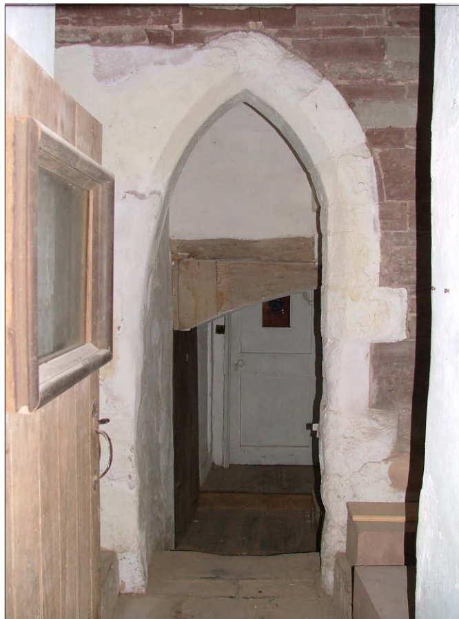
Plate 6: Door D18 Leading from ground floor room to base of main staircase
