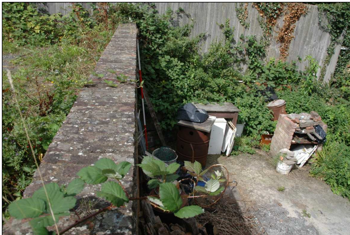
Plate 12: Retaining wall at the eastern end of the car park (looking north)
