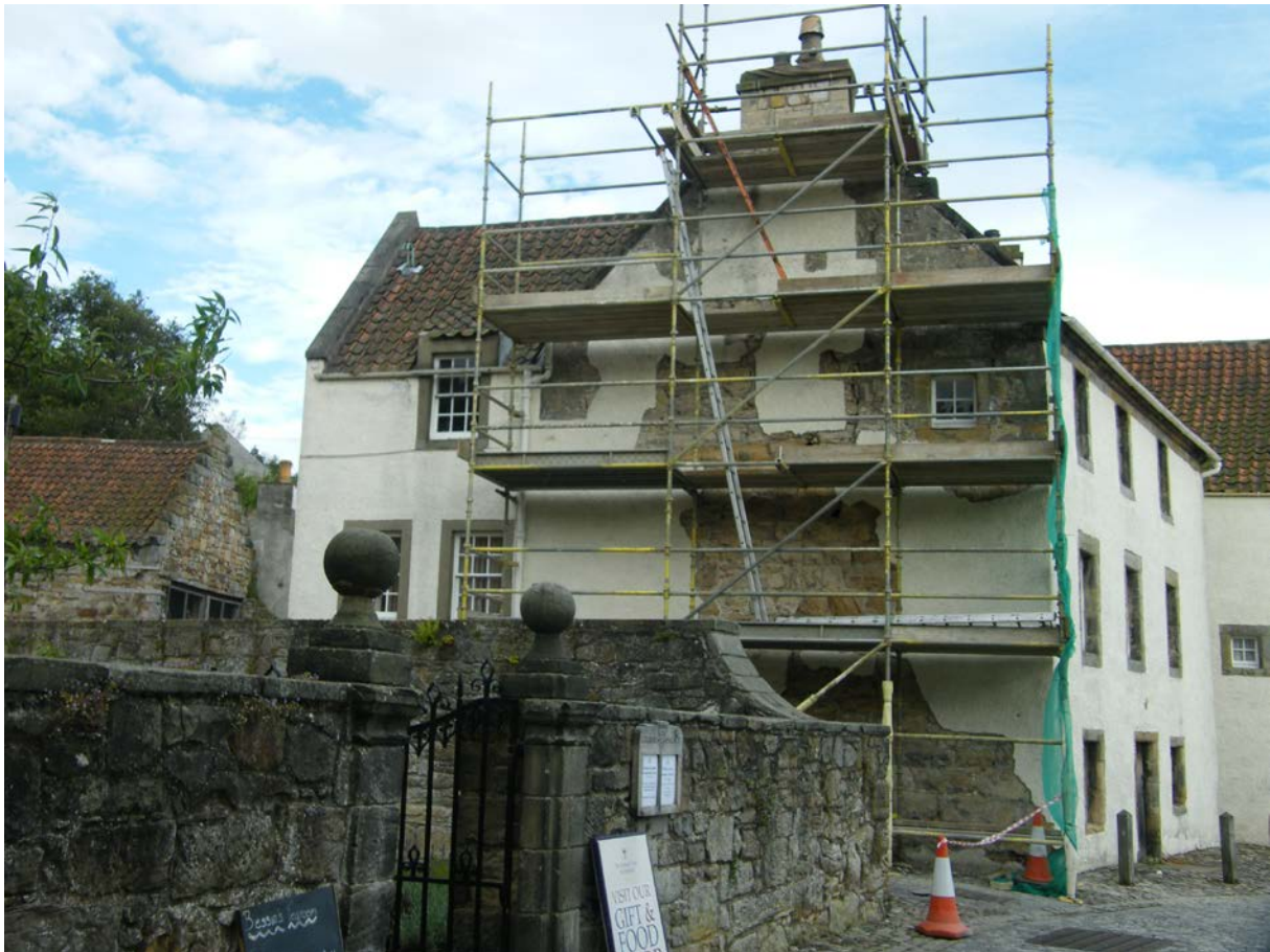
Sandhaven West – Gable under exposure
