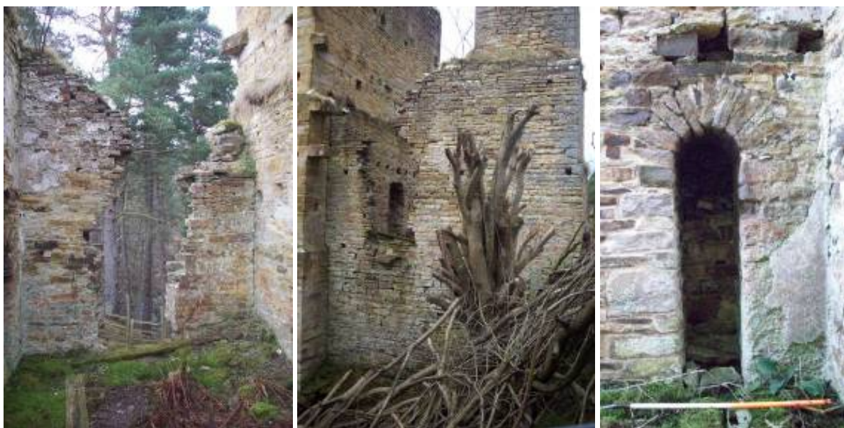
Plates 6, 7 and 8: Interior and exterior of east gable and access to chimney
