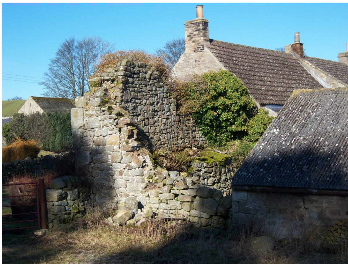
Plate 6.27 General view of the western gable wall of the early range from the SE
