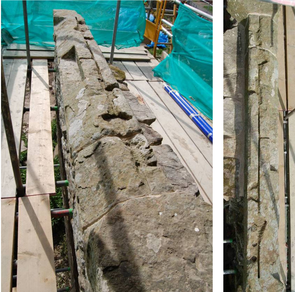
Plates 4.10 and 4.11 South wall of chapel, first floor – detail of window sill stone
