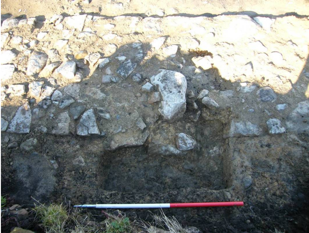
Plate 6.2 evidence for pilaster buttress, south wall of early range (N at top)
