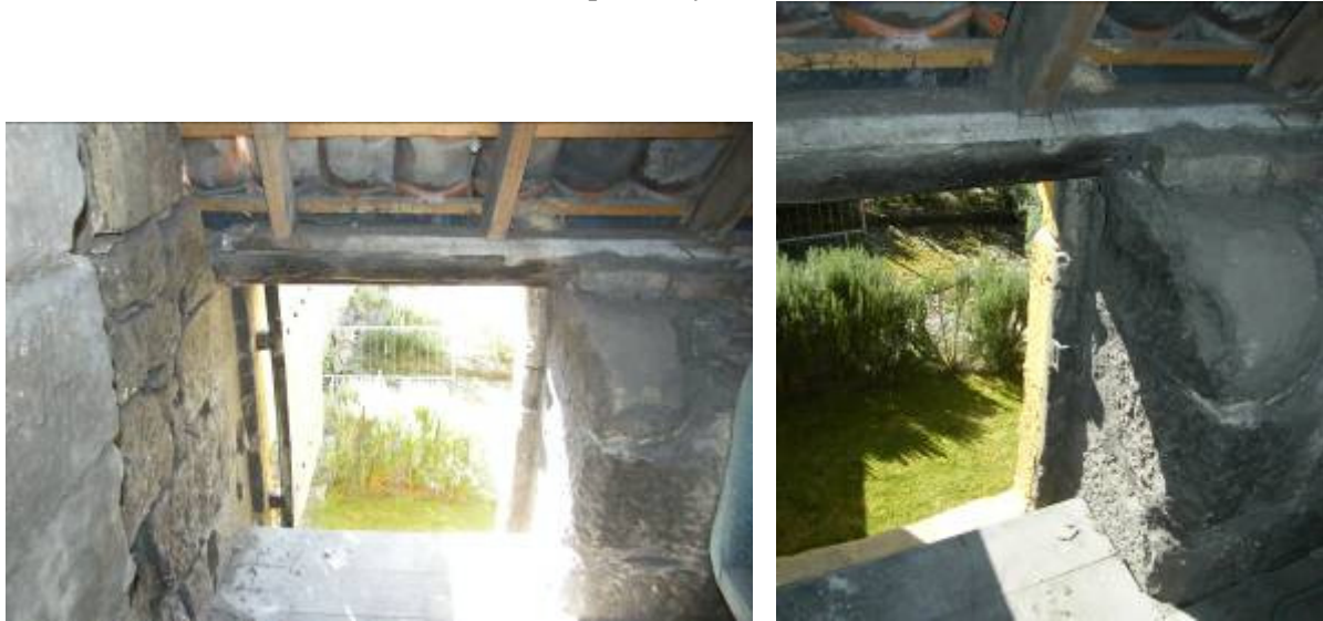
Figure 24 – Evidence for a much taller opening into loft of E extension.
