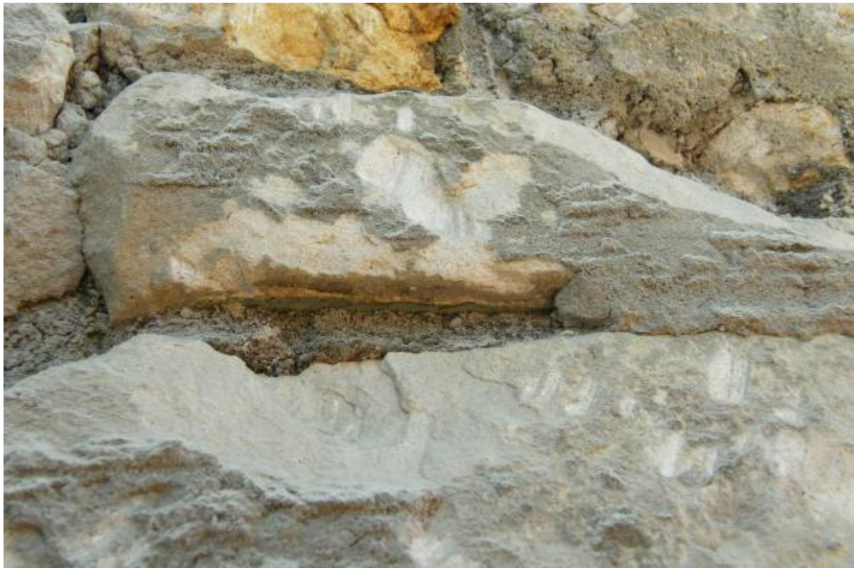
Figure 27 – Remains of painted plaster on the underside of stones used for the flue repair and blocking of fireplaces (017, 018, 024 – here 017) of the W gable.
