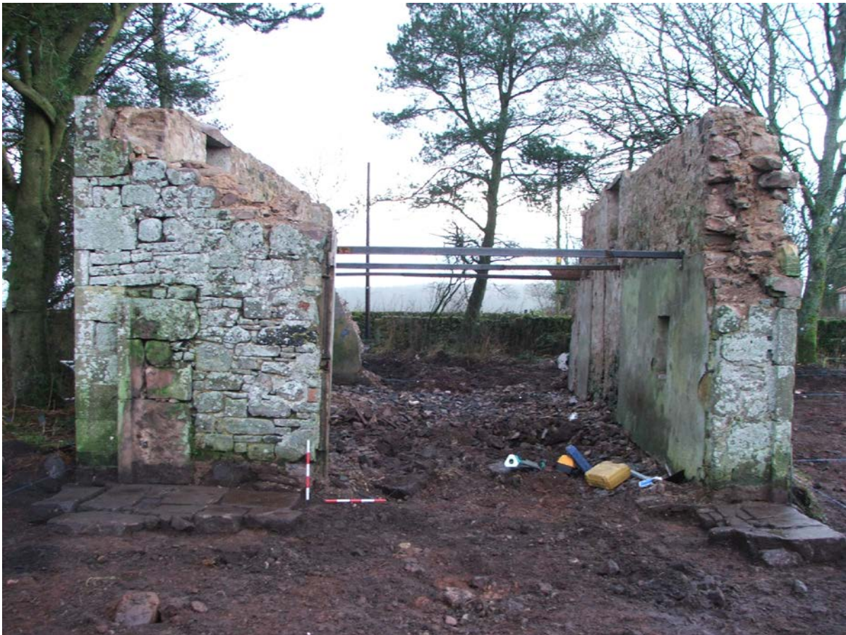
Plate 6 Post excavation of eastern area (Photograph 060) with surviving doors and threshold stones exposed; general view from E (0.50m scales).
