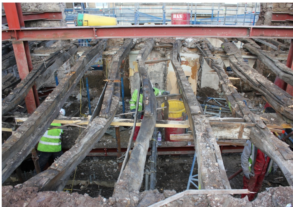
Plate 1 Group A Joists of crooked and branched oak revealed in 1 st floor ceiling; potentially a very rare native oak structure of late medieval or early post-medieval date. Relicts of Jed Forest perhaps?
