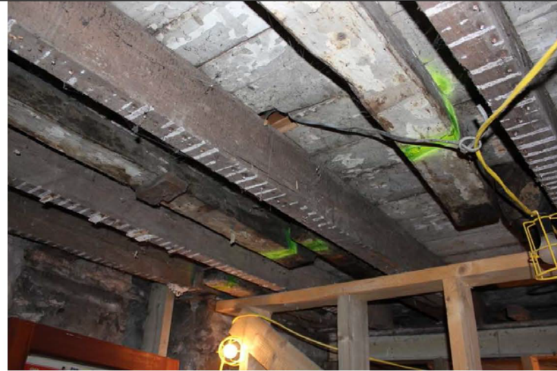
3 Hewn, roughly square conifer joists in ground floor ceiling (in between more regular rectangular joists assumed inserted later) running from the main block forward into the front extension at the NE side of the central pend. Photo: C Mills
