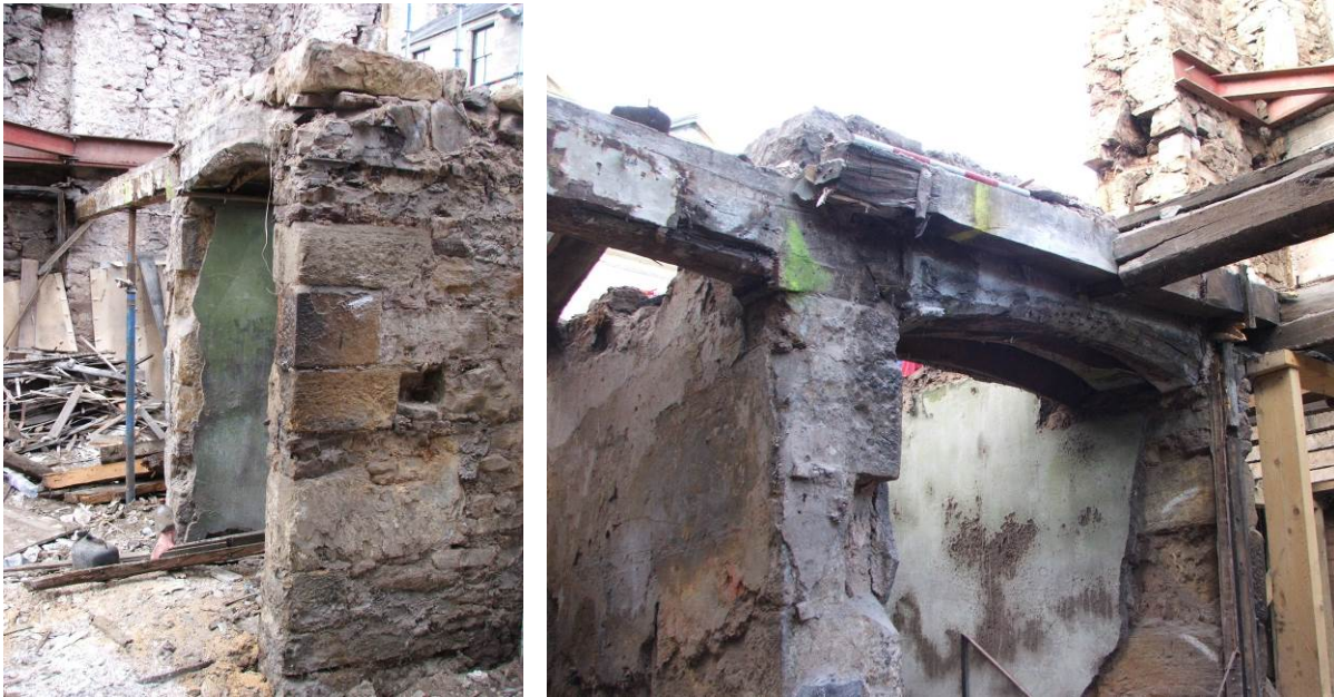
Plates 9 and 10 Pend walling showing timber arch; a remaining early principal joist 063 can be seen beyond to the left
