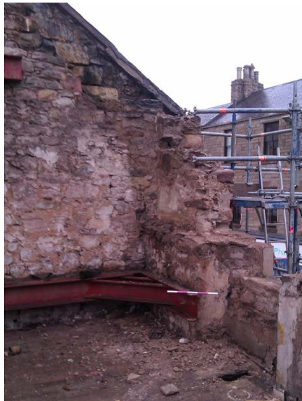
Plate 6 SW end of the frontage wall, interior at second floor level, showing the internal off-set; note also the embedded crow-steps and gable head in the adjacent SW wall; looking west
