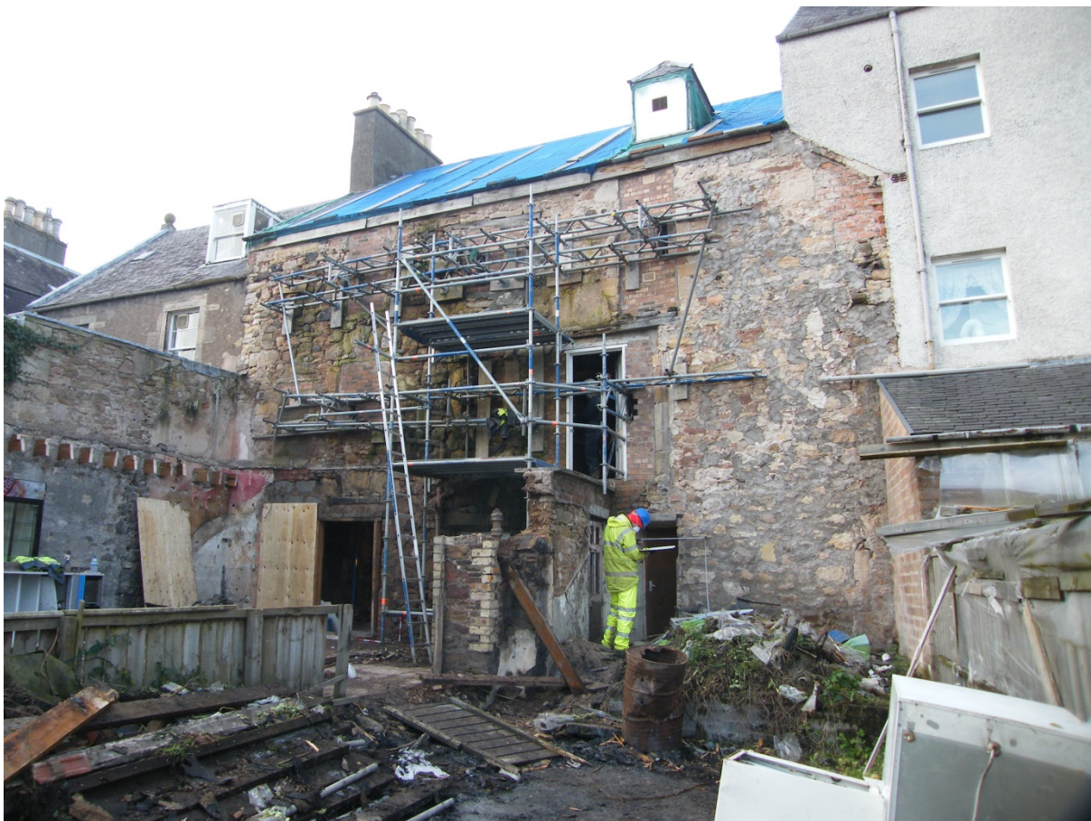
General view of the rear of the property during early stages of demolition
