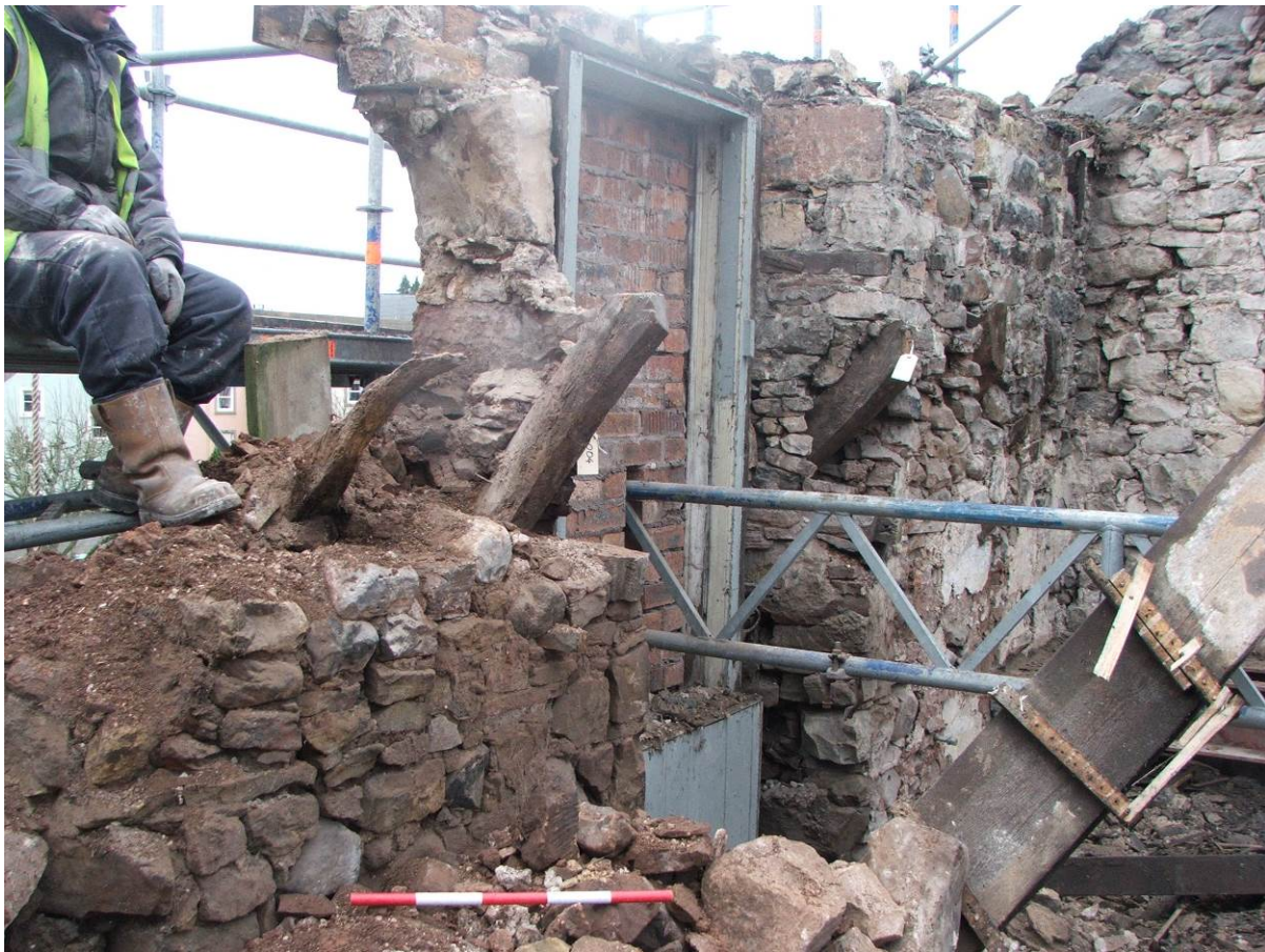
Plate 21 The rafter foot assemblies as partially exposed during early stages of demolition
