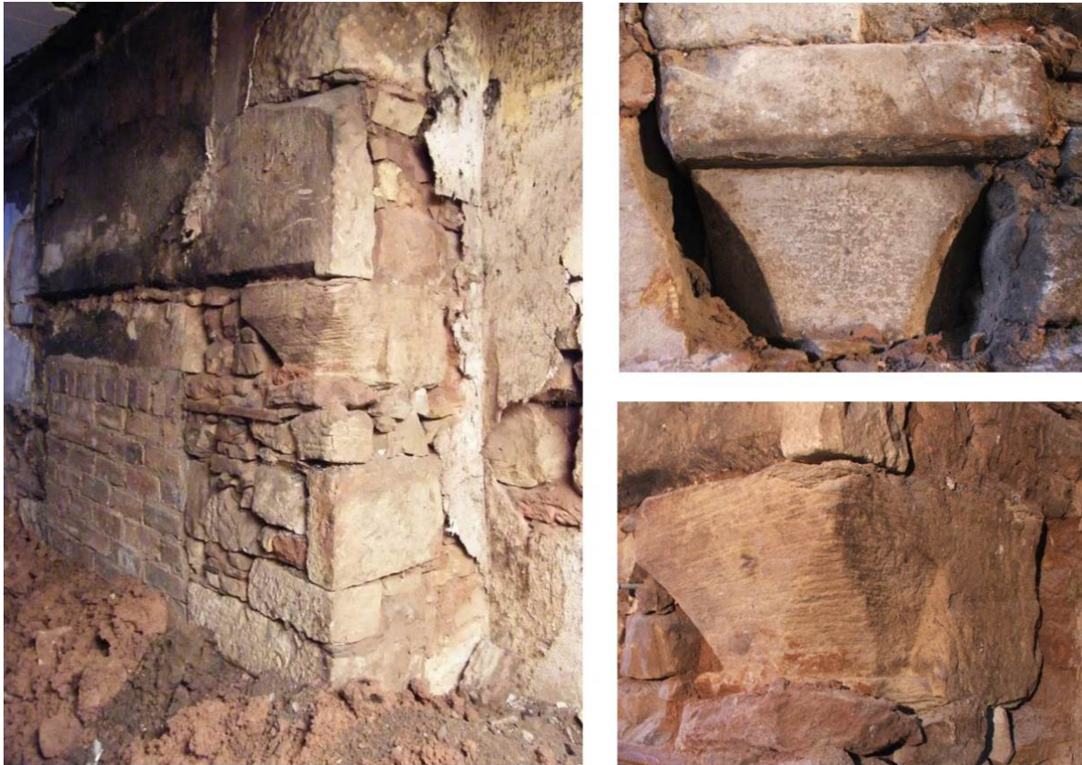
Plate 36 Lower stage of the chimneybreast within SW gable wall (074), showing extensive use of recycled architectural stonework, including the substantial lintel (085)
