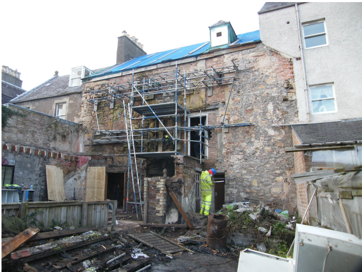
General view of the rear of the property during early stages of demolition
