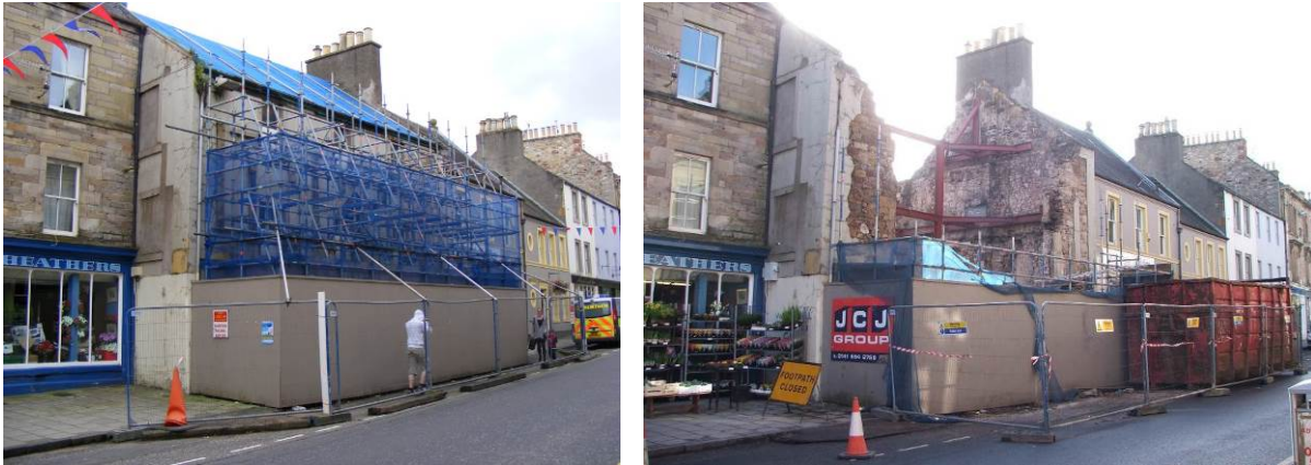
Plate 1 Following propping in 2012 – street frontage, looking south (Demolish31HighStreetJedburgh web-site) Plate 2 Demolition nearing completion – the street frontage, looking south
