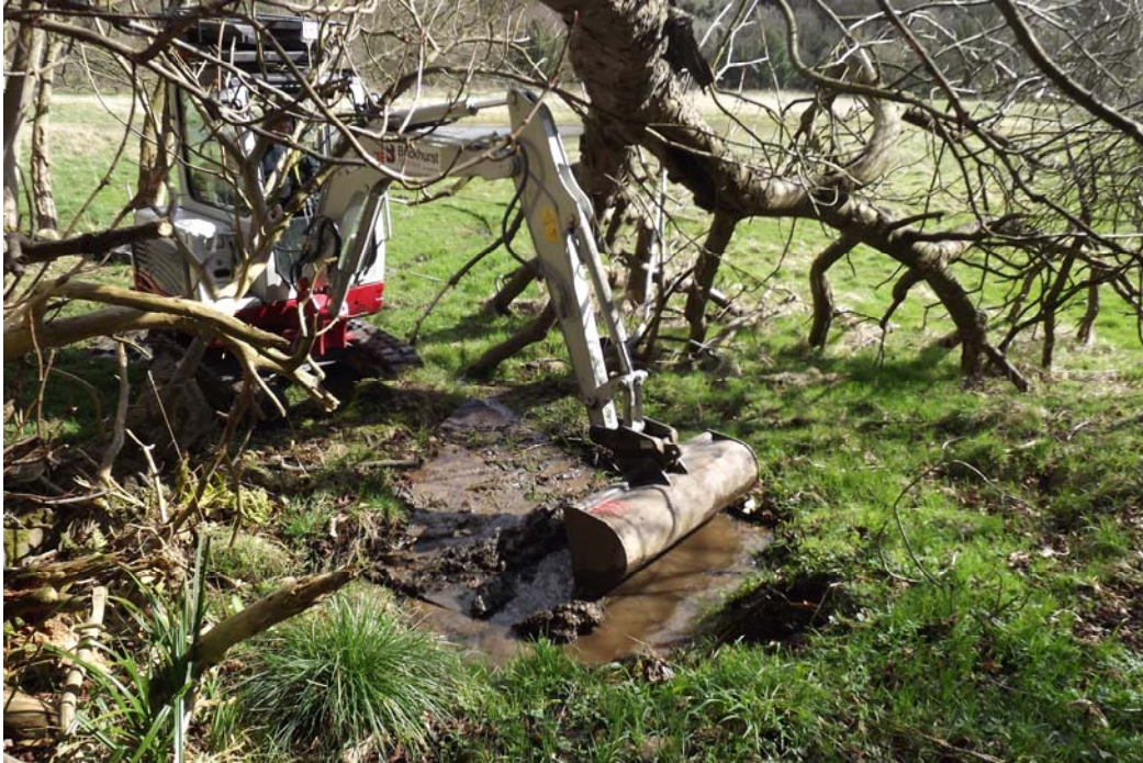
Plate 3 Removing the Fe plate from atop the brick lined drainage feature (Photograph 037)
