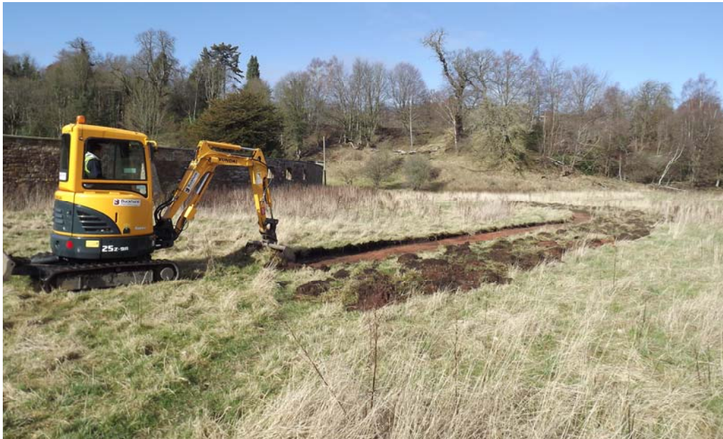
Plate 2 Working shot looking west. Note the red blaze (107) being revealed across the route of the path (Photograph 015)
