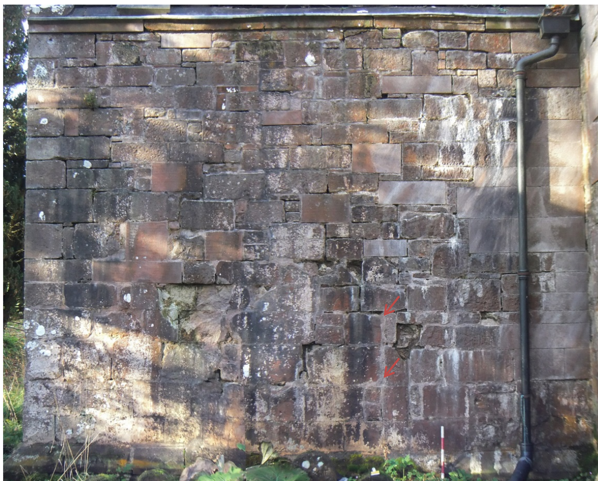
East exterior wall of the south transept before commencement of conservation works; the red arrows indicate the south jamb of the secondary entrance
