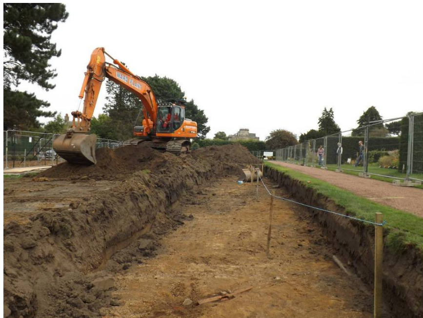
Plate 1 Mid-ex photo of main excavation area showing topsoil (001) and sandy clay subsoil (006), (photo 020).
