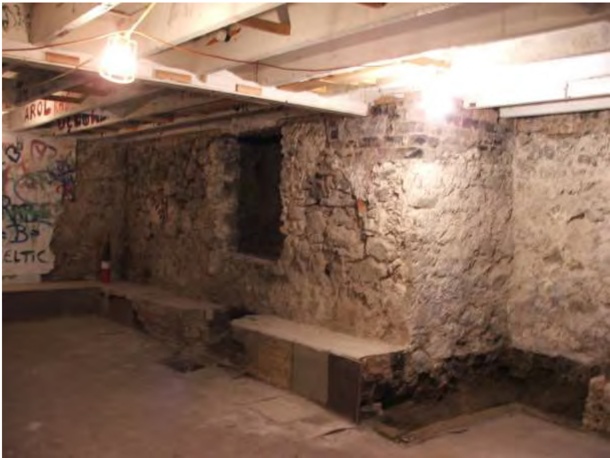
Plate 4 Wall stub 151 within the SW part of the basement (Room 1), looking SW
