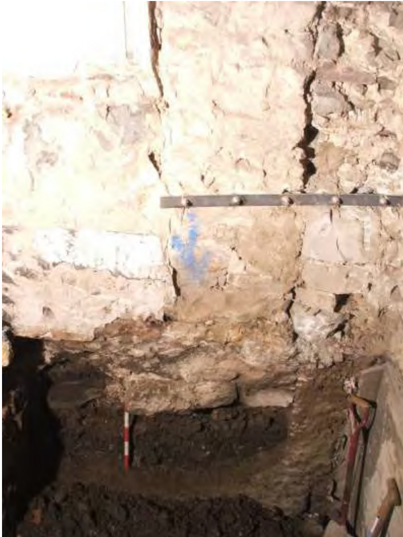
Plate 2 North wall of Panmure House at basement level, northeast corner. 1690 masonry to left and reduced masonry of boundary wall to right; the vertical butt joint between the two can clearly be seen behind the metal strap; also visible in section below are cultivated soils on the west side of the boundary wall; looking north
