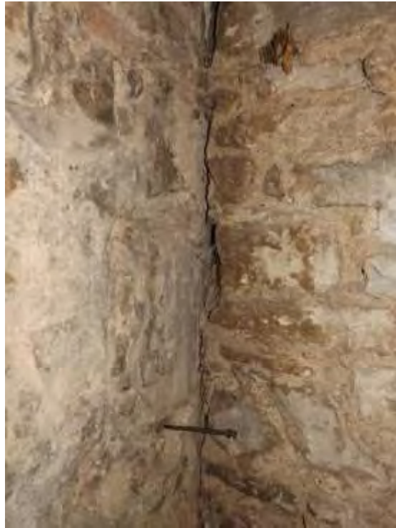
Plate 5 thin render/plaster, 173, on face of main range (left) trapped behind eastern jamb (right)
