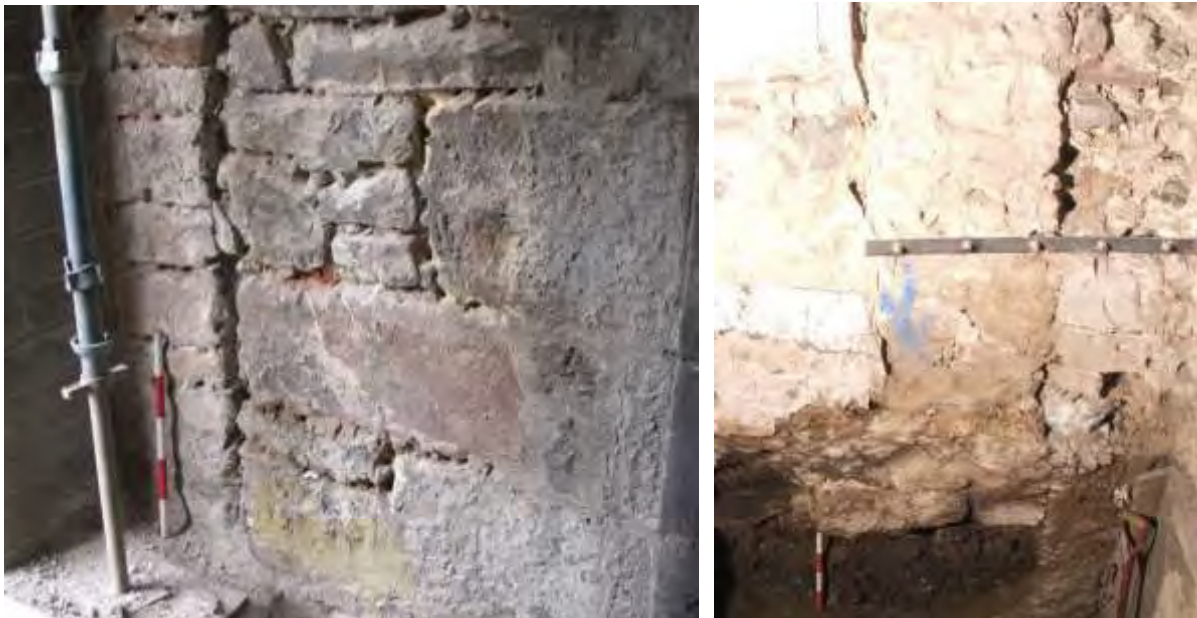
Plate 20 jamb 240 exterior looking east; Plate 21 jamb 240 interior looking north (jamb to left of metal strap)
