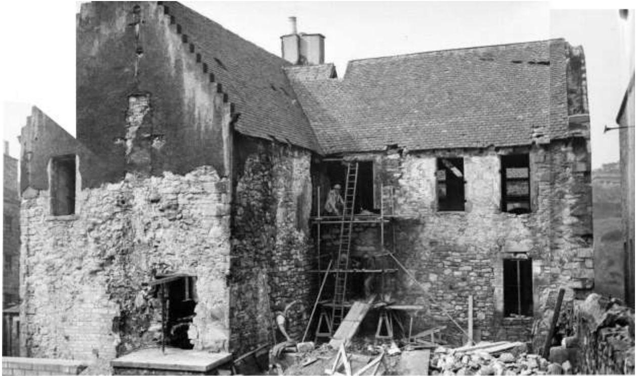
Plate 16 composite photograph of 1950s works showing south elevation works of 1956-7 in progress (SCRAN / The Scotsman)
