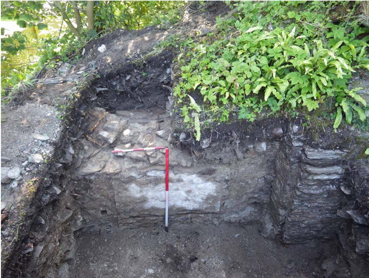
Plate 2 West (interior) face of wall [104], joined to wall [108] by slate pinnings; wall plaster relating to the later press can be seen behind the vertical scale
