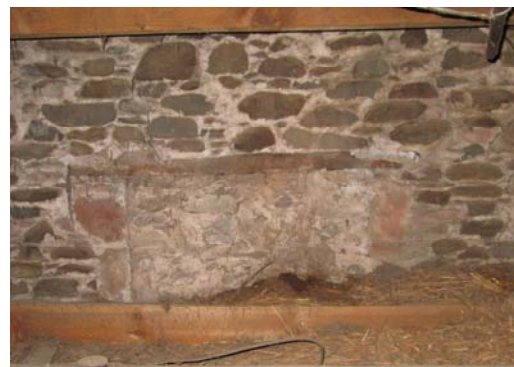
Plate 7 Blocked attic window interior (155)
