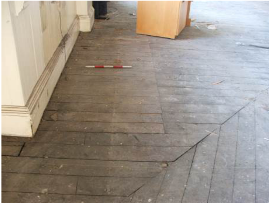
Plate 9 Rectangular patch in the floor in the area of the former stairwell
