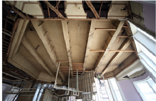
Plate 6 Panorama of evidence in the roof for the former octagonal lecture room
