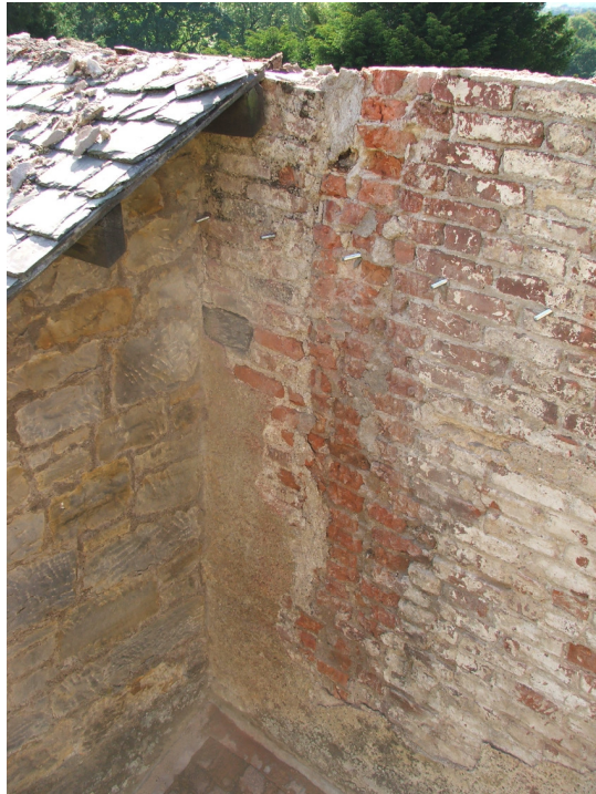
Plate 5 exterior stub of 010 clawed back flush (mid frame) and infill 024 brickwork to left behind later lean-to
