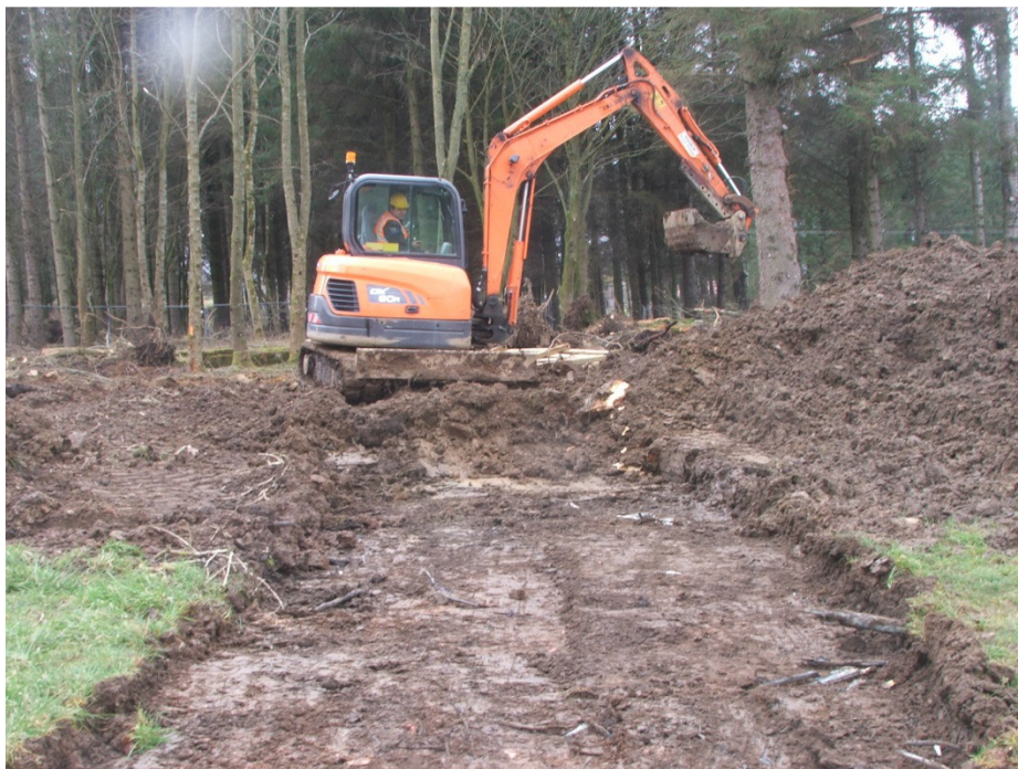
Plate 1 Path under excavation. Building [1004] can be seen to the rear of the machine, behind the trees.
