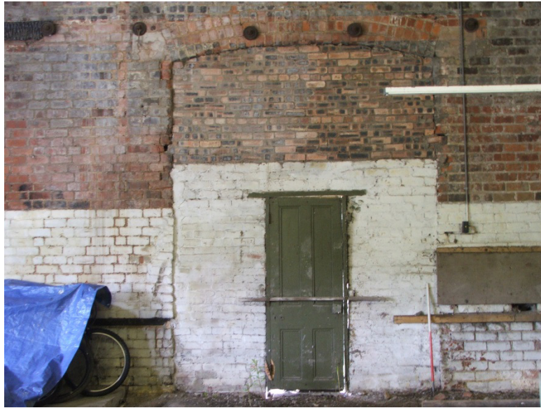
Figure 16 Internal north wall showing blocked archway and inserted door; openings in the brickwork to the right of the door indicate the position of the loading platform.
