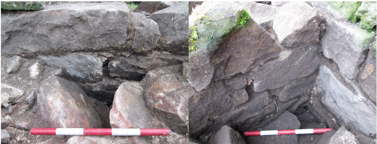
Plate 2 Trench 1. Detail of east face of east wall of Engine House 1, Wall [100], showing the wall line continuing to the north, beyond the collapsed return with the north wall of Engine House 1.
