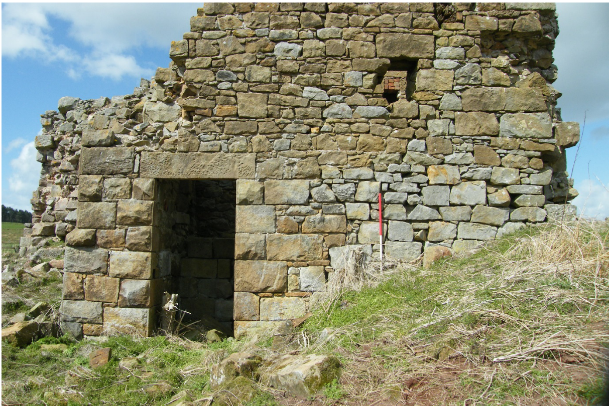
Plate 4 Engine House 1 east wall [100] showing earlier construction phase of grey angular blocks in its northern extent. Facing west..
