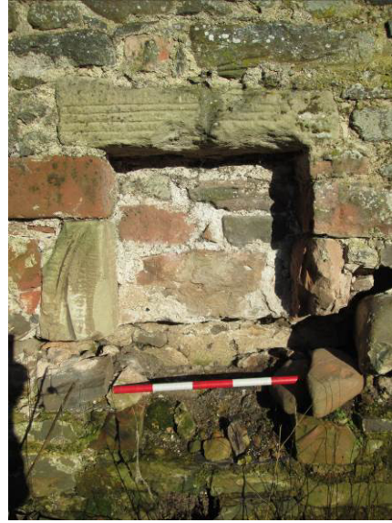
Plate 4 Mark from wheel on sandstone jamb (photo 202)
