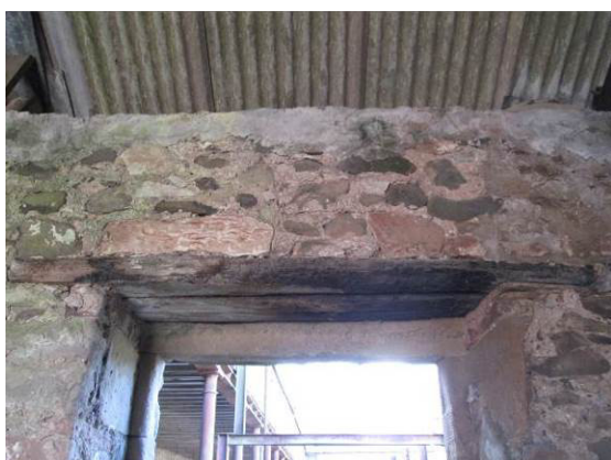
Plate 15 Charred lintel above door east range (photo 194)
