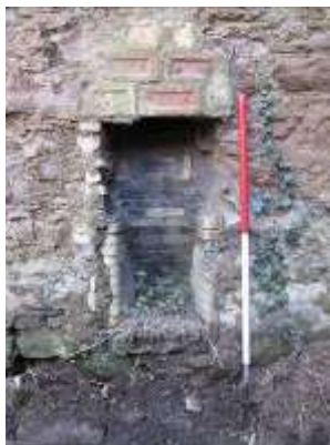
Plate 7 Rough inserted fireplace
