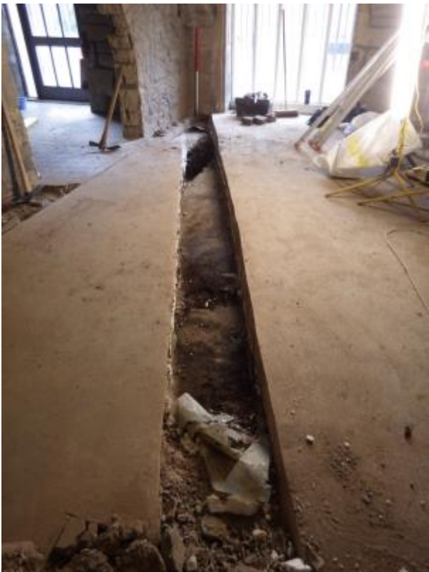
Plate 13 ST3, general view of initial breaking out with previous service track visible in b/g. Facing N
