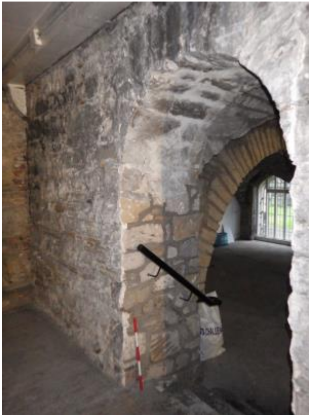
Plate 77 General view from undercroft to crypt at David Boyle Lair with cut-through round-headed door. Facing south-east.
