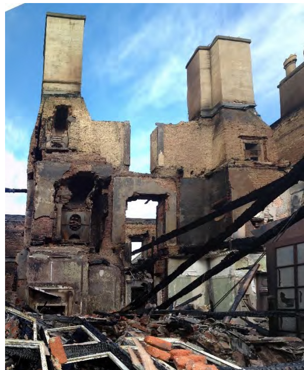
Plate 12 composite photograph of central spine post-fire
