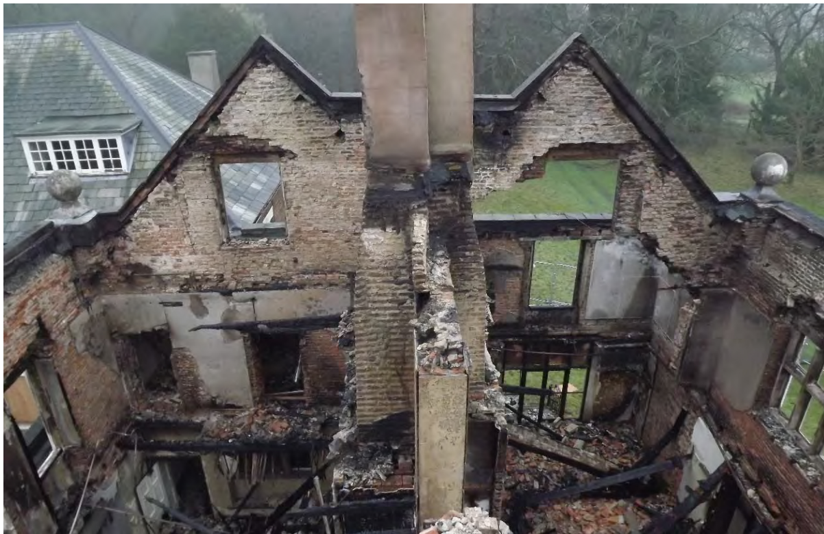
Plate 10 east gable post fire pre collapse /demolition
