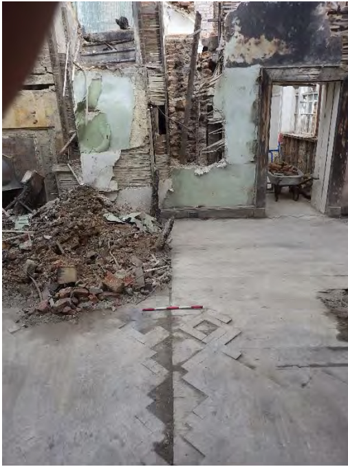
Plate 70 room G09 shows earlier flooring to west stopping on line of former gable
