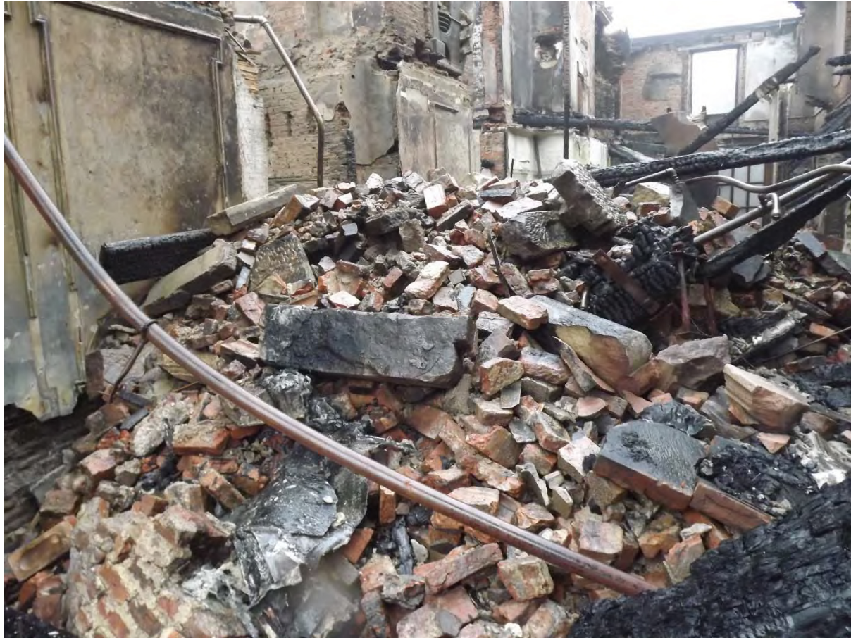
Rubble collapse within Woolsington Hall
