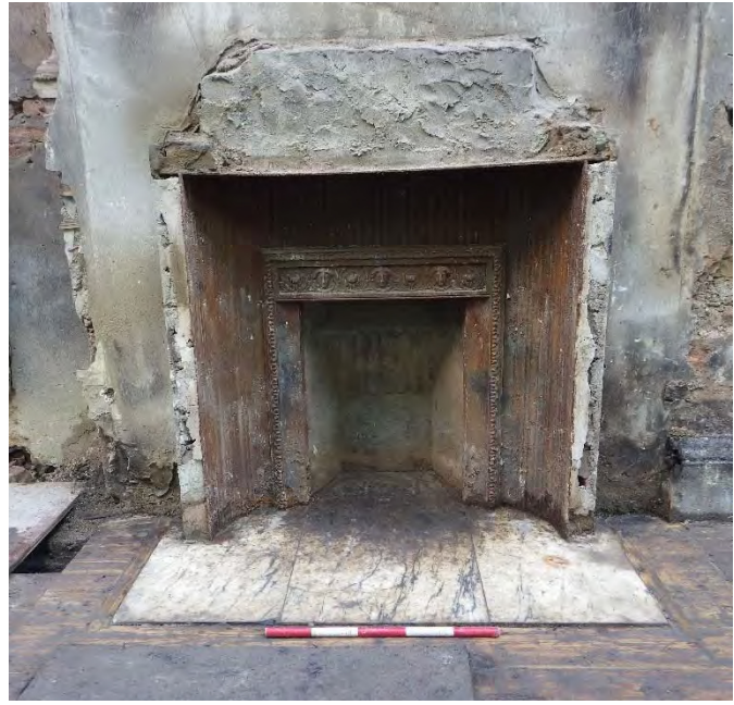
Plate 58 G03 fireplace post fire
