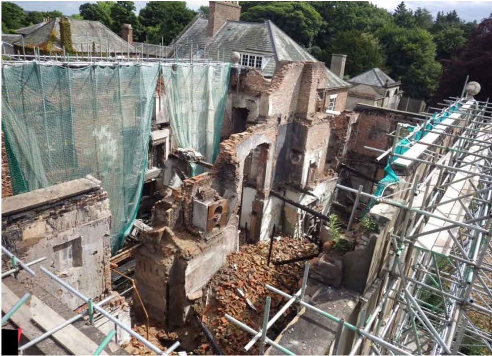
Plate 13 The masonry of the spine wall after the first stage of demolition
