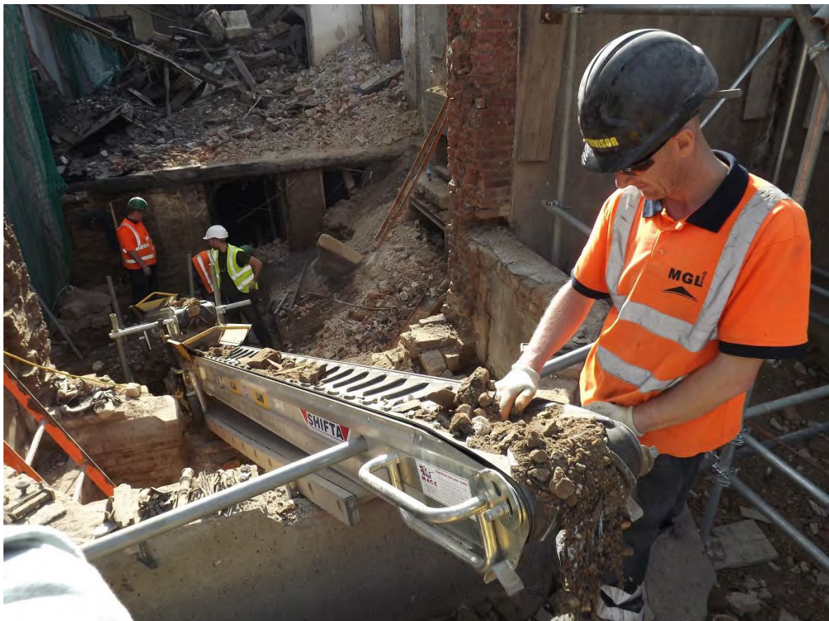
Plate 8 Inspection of debris on conveyor-belt, excavated from within the basement area, July 2016
