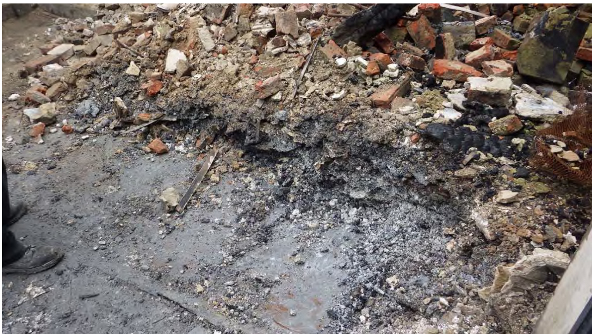
Plate 55 Ground floor flooring with the burnt remnants of the structure above reduced to 30 cm of ash
