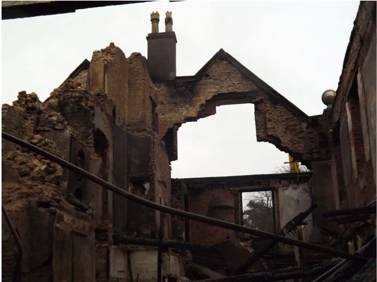
Plate 5 South-east gable before demolition on 9 January 2016, illustrating its perilous state
