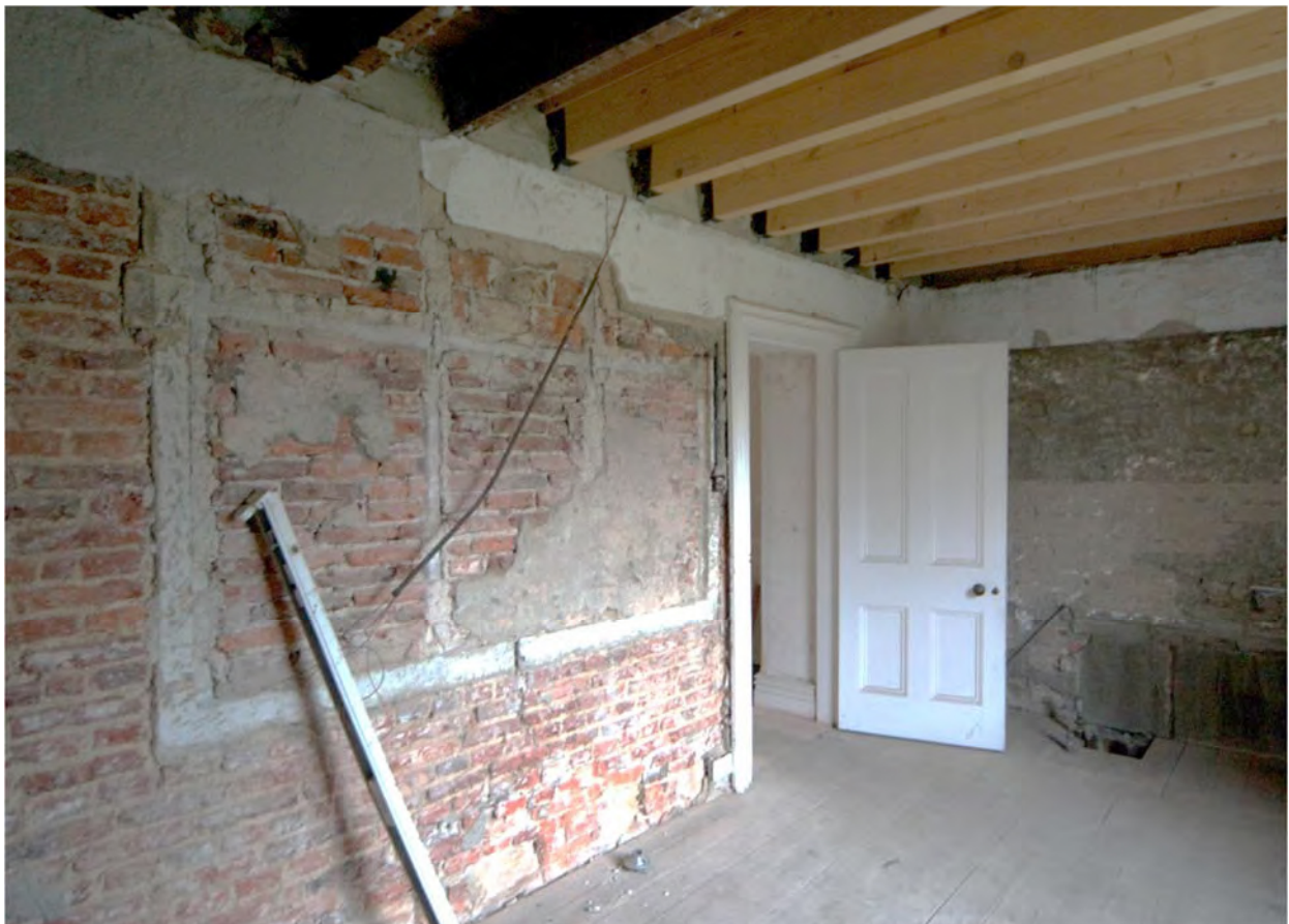
Plate 38 The former window within the west wall of Room F04, as seen in situ before the fire within room F5 (find no 097)
