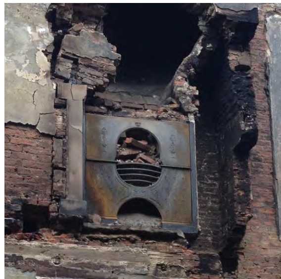
Plate 35 room F04 fireplace and surround in situ post fire
