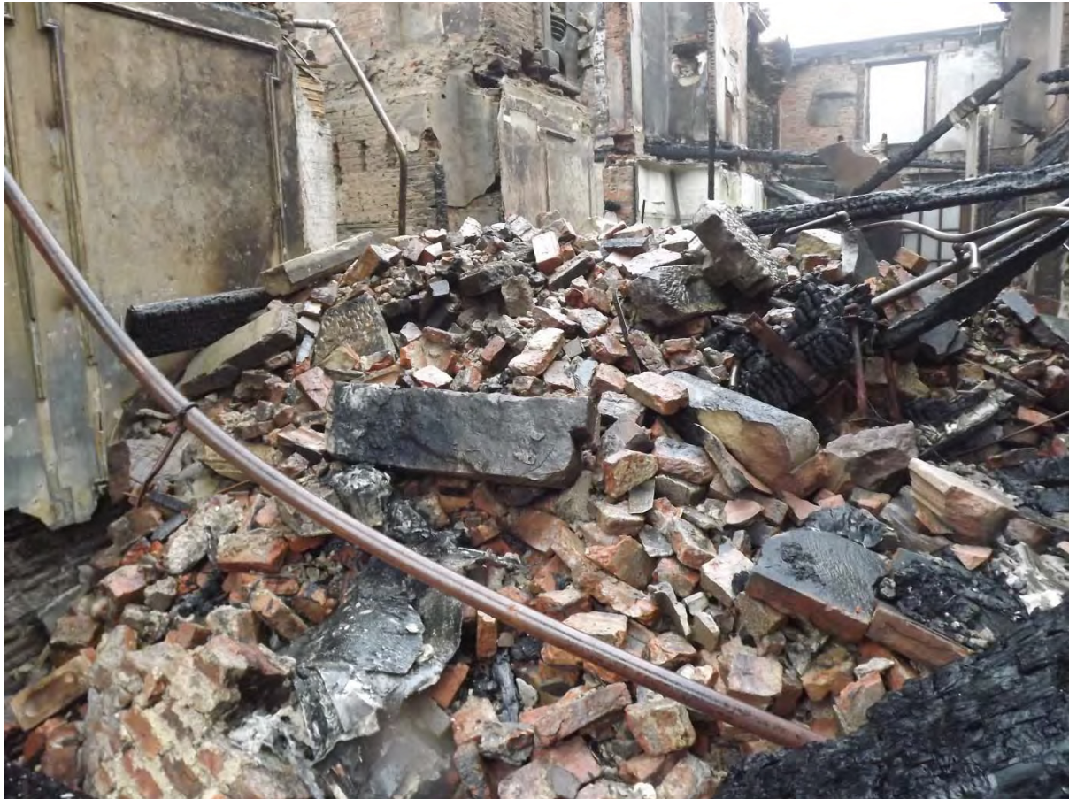
Plate 15 Rubble collapse within Woolsington Hall
