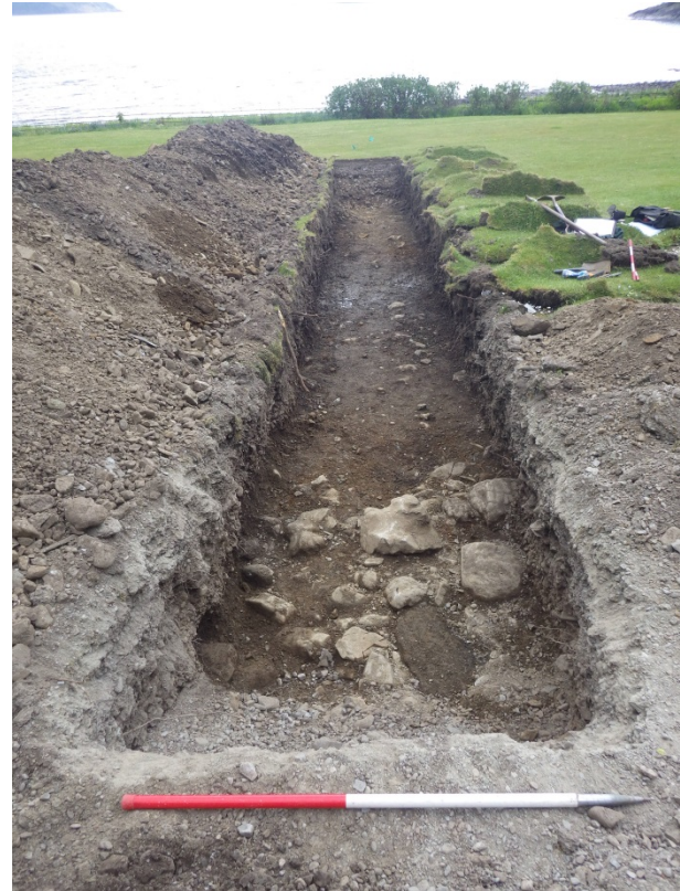
Plate 12 Trench 4, general view post-ex with asphalt [404] and stone concentration [405] in foreground. Facing south
