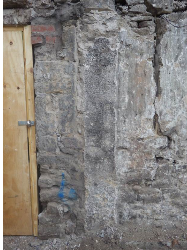
Plate 14 Stair tower demolished showing tower masonry built over blocking of window 166 and survival of former historic harl
