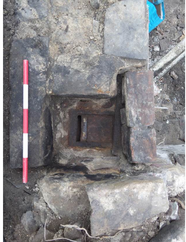
Plate 9 South elevation of lean-to detail of flue emptied shows flue damper in situ and partially open
