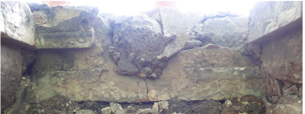
Plate 18 View up to lintel remnant, shows imprint of window case, one bar hole and a possible glazing groove
