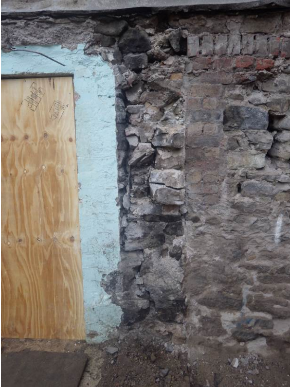
Plate 13 Stair tower demolished showing tower masonry built into window 171 with a little historic harl in situ below the window
