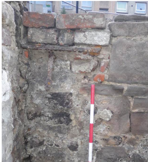
Plate 10 Wall face of flue shows damper handle (bent over) and bricked up opening below?
