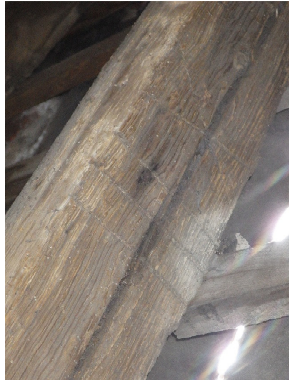
Plate 8 Truss 9 rafter 025 cut no 079
