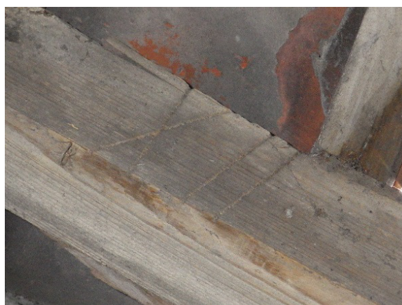
Plate 22 Truss 4 rafter 010 cut number "XII" 059
