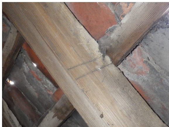
Plate 12 Truss 11 rafter 029 cut number "II" 084
