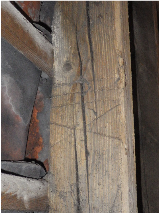
Plate 7 Truss 9 rafter 024 cut no 078
