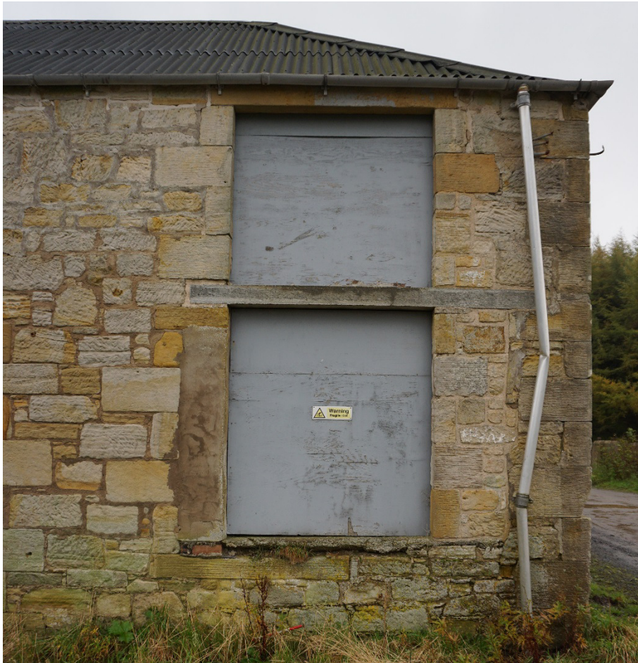
Plate 12 Building 3 NW elevation original window 47 bottom left cut by later opening
