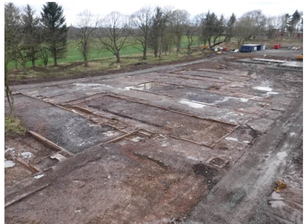
Plate 50 Building 86, Rooms D (left) and H (right) with Building 22 in background. Facing NW
