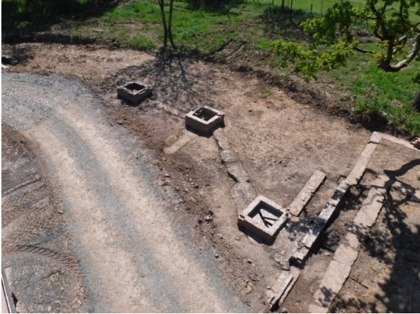
Plate 77 General view of junction boxes [323] (left), [324] (centre) and [325] (right) south of Building 24, at right. Facing SW
