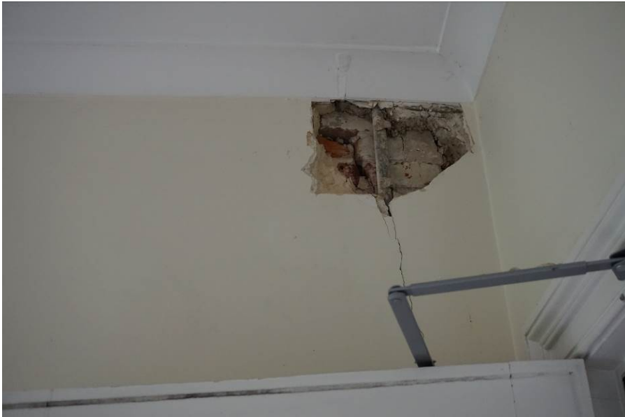
Plate 2 room G.05 wall plaster removed around crack
