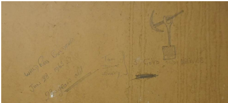
Plate 12 room F.01/F.04 partition graffiti
