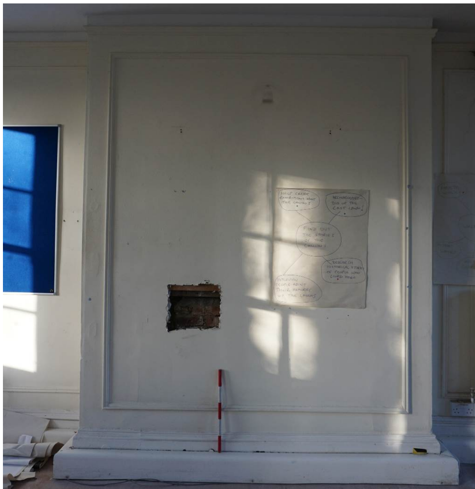
Plate 1 room G.04 brick blocking of fireplace exposed
