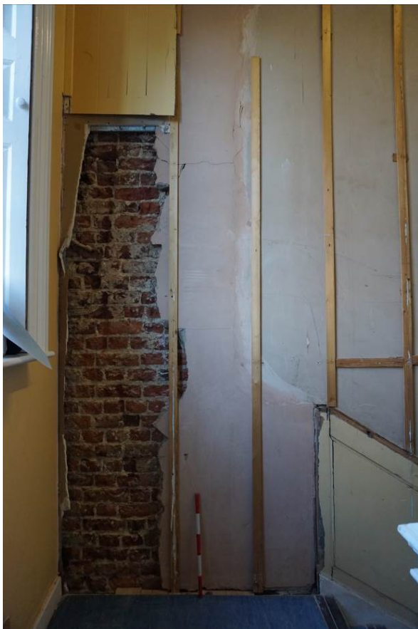
Plate 7 room F.01 elevation showing multi-phase repairs of south elevation
