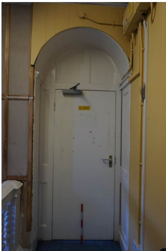
Plate 18 room F.01 door to F.02, note secondary arch over door off centre
