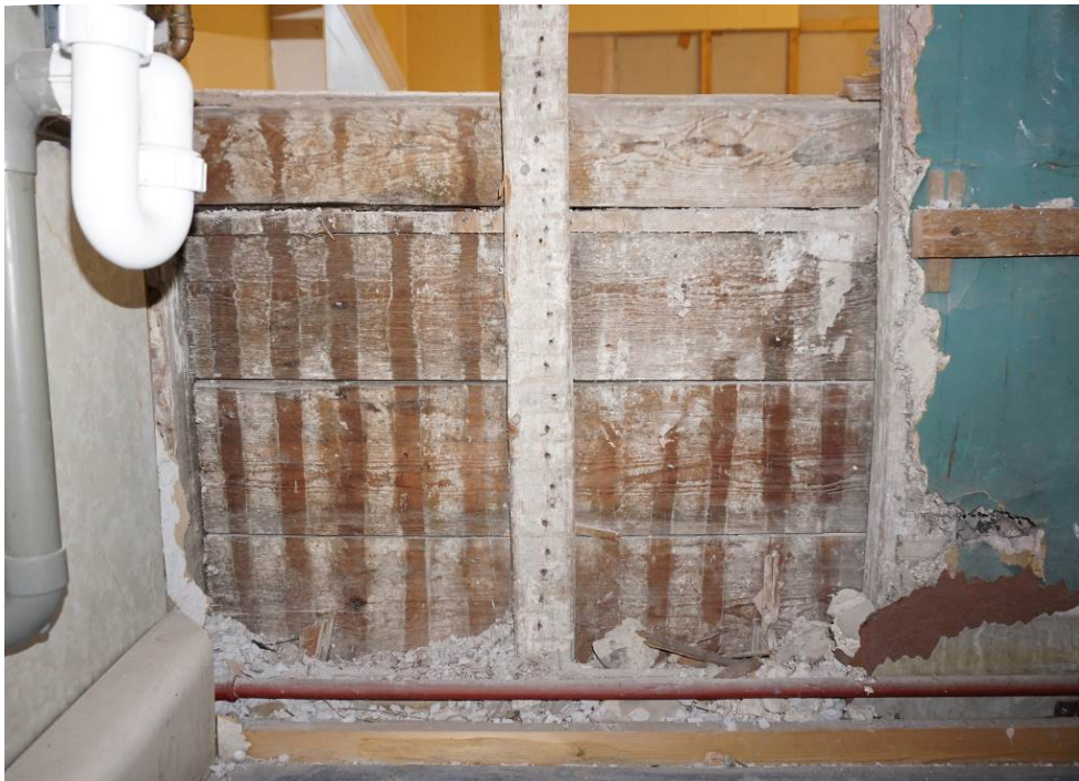
Plate 16 rear of partition showing rear of panelling and neat lime washed studs
