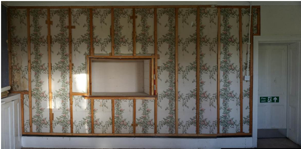
Plate 4 room G.06 floral wallpaper exposed
