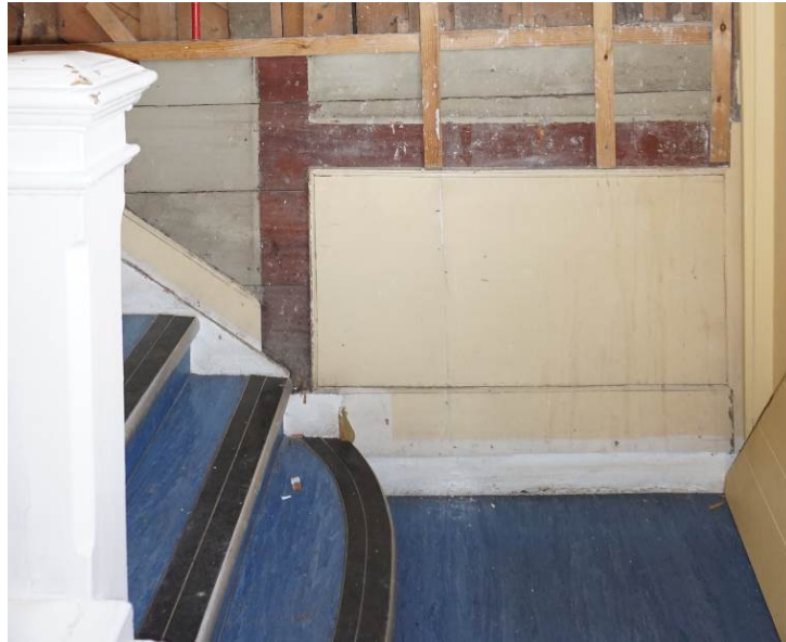
Plate 11 half landing showing bowed step and deep skirting beyond
