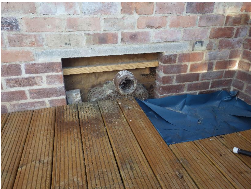
Plate 3 glasshouse boiler opening into glasshouse, looking north-east
