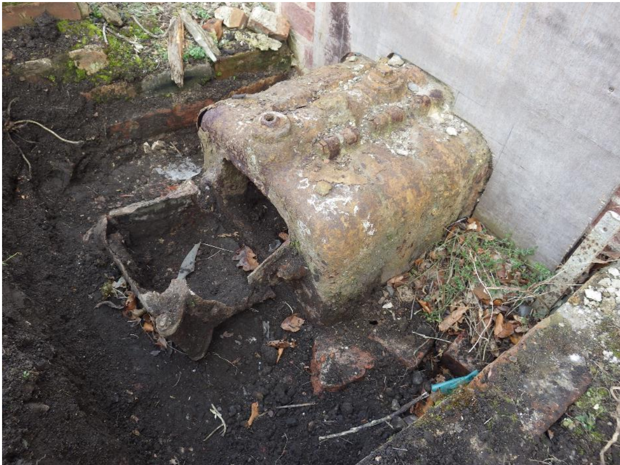
Oblique view of the Beeston Junior Boiler, incorporated within the wall of the glasshouse.
