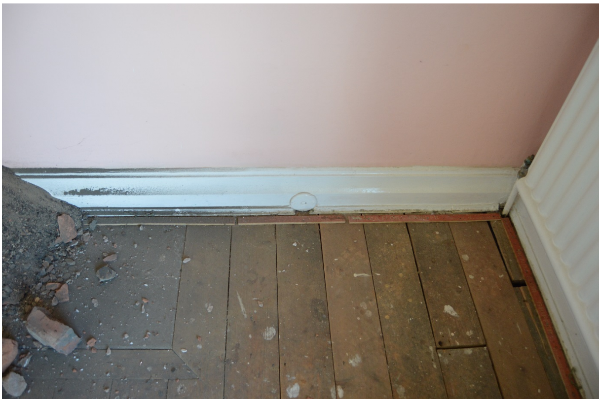
Plate 15 Example of lapsed electrical fitting, bedroom 2 (photo 331)
