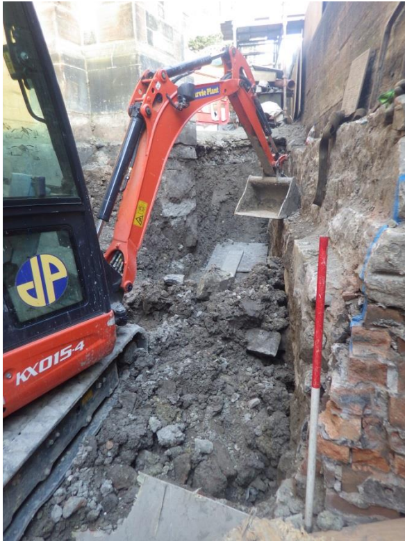
Plate 27 View of excavations southern courtyard, school building to N, retaining wall to S
