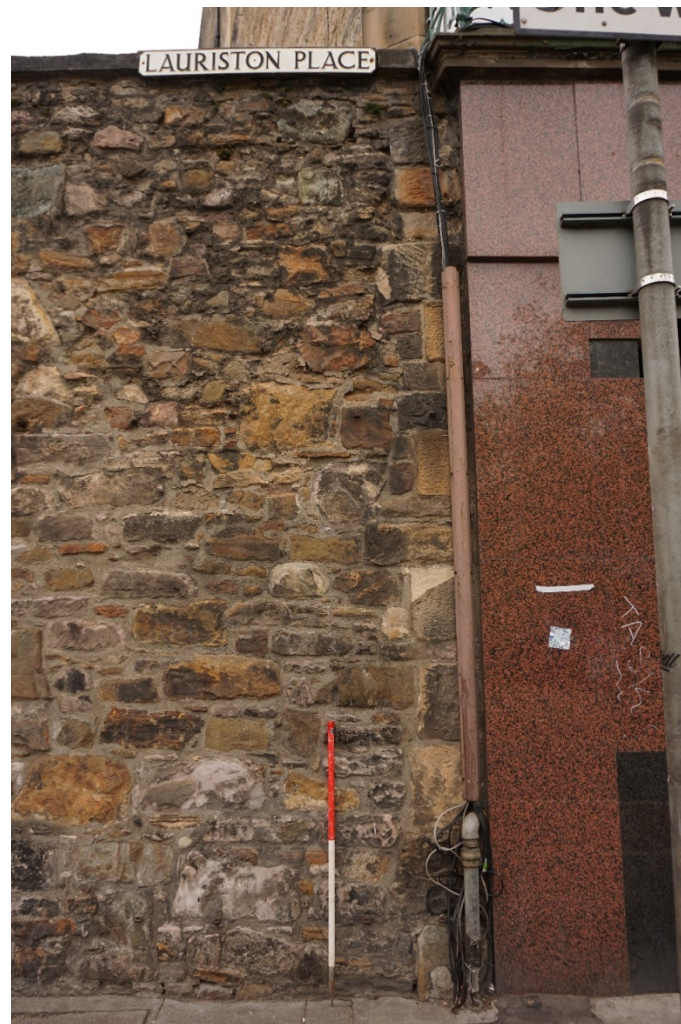
Plate 1 Eastern Extent of the Telfer Wall, at the junction with No 61 Forrest Road
