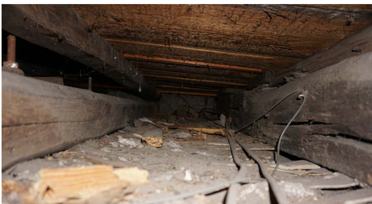
Plate 3 joists 2 and 3 to left and joist 4 to right, note bolt in joist 3, looking south (photo 23)
