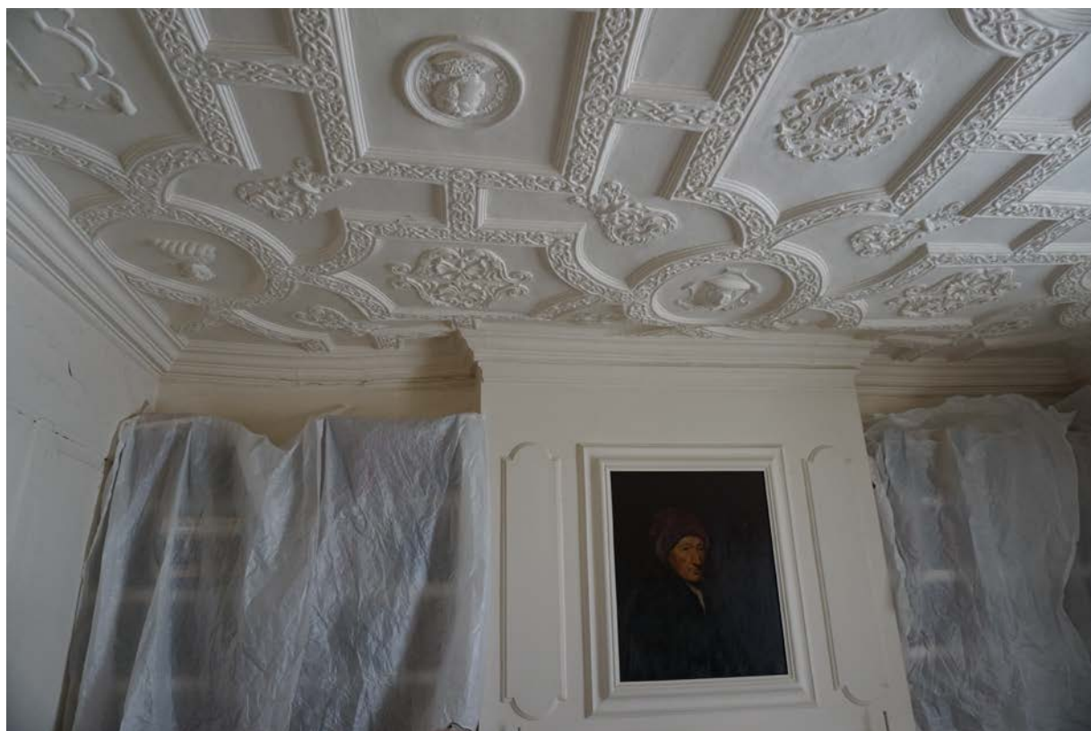
Plate 1 early 17th C plaster ceiling of library slumping above fireplace (photo 01)
