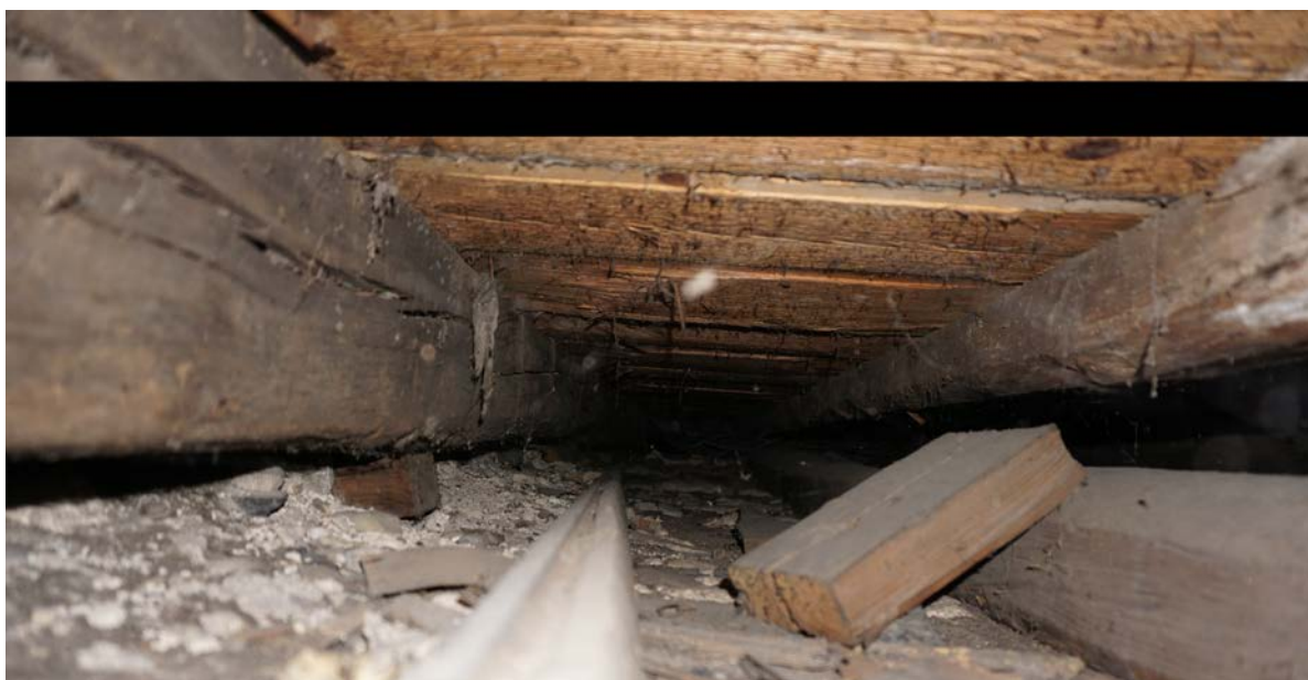
Plate 8 joists 14, 13 and 12. Joist 14 to left, 12 to upper right and 13 to lower right.
