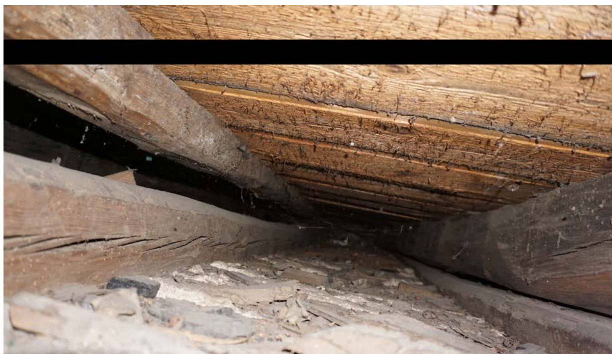
Plate 7 joists 10,11,12 and 13, joist 10 to upper right, joist 11 lower right, joist 12 top left and 13 bottom left, looking north (photo 45)
