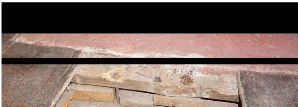
Plate 9 bolt from plaster ceiling below joining joists 2 and 3 with timber packing between joists
