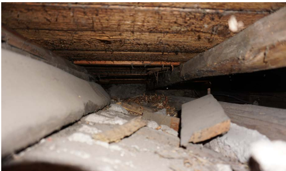
Plate 2 joist 2 and 3 to right, 2 at top 3 at bottom showing gap between and bolt from below, joist 15 to left looking south, note sloping of plaster below (photo 22)
