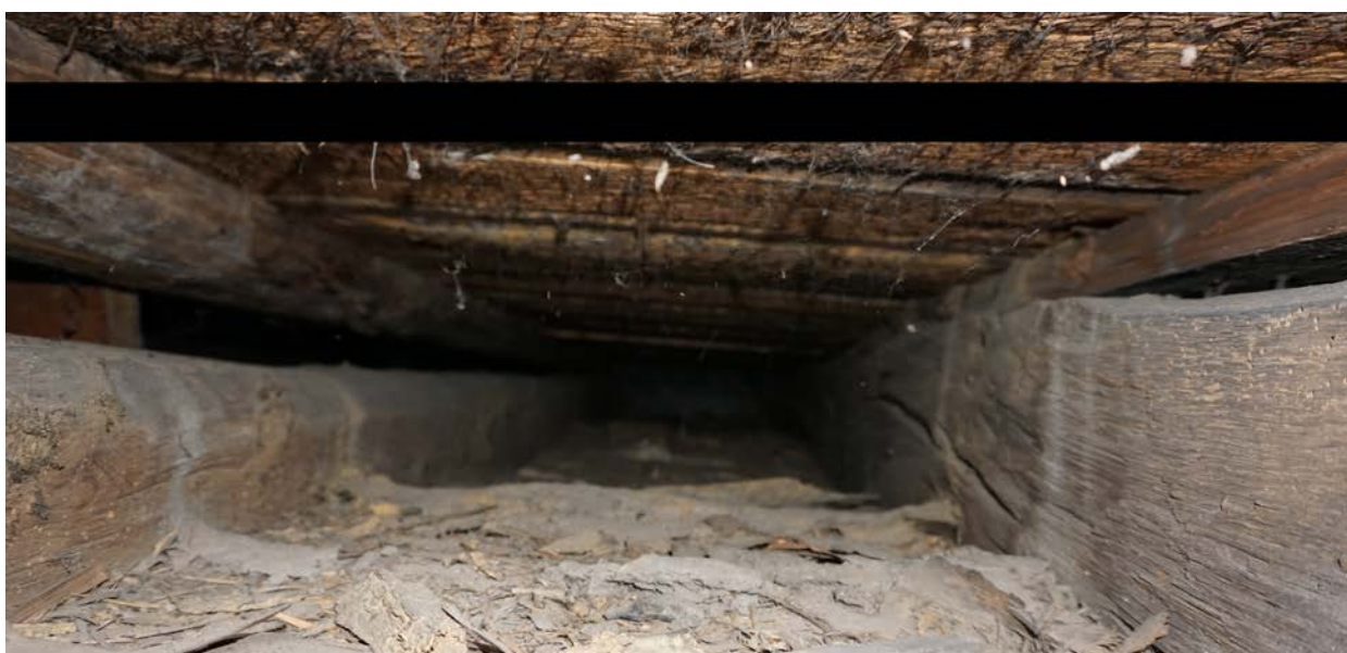
Plate 6 joists 7,8 and 9, joist 7 to right, joist 8 top left and 9 bottom left looking north (photo 40)
