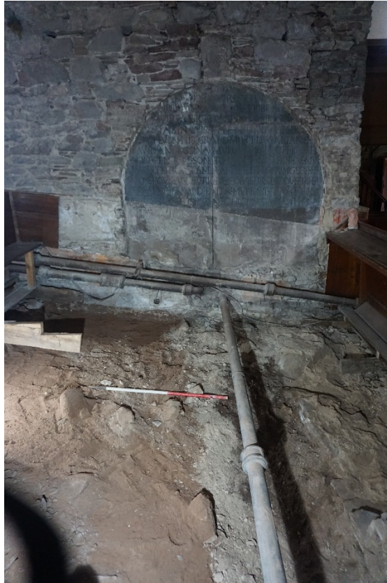
Plate 8 Demolition rubble (003) over graveyard soil (002) and red sand ramp (004) to the left.
