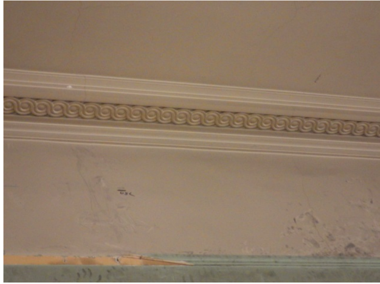
Plate 30 Room G.194, guilloche crown moulding detail
