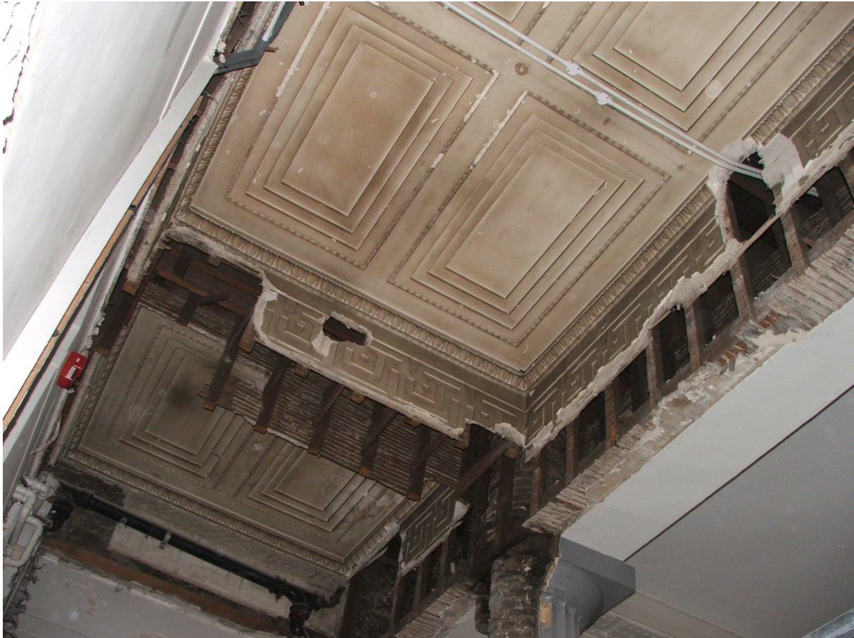
Plate 18 G.Z27 general view of ceiling structure with relict partitions showing egg-and-dart and Greek key crown mouldings
