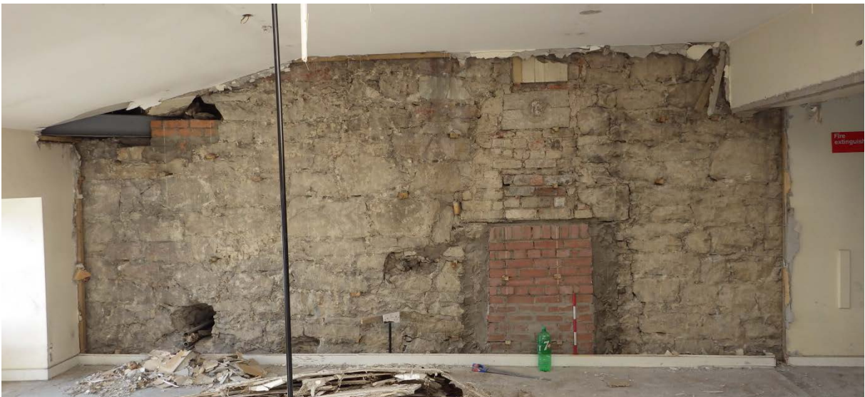
Plate 57 Room 2.368 south wall with historic fabric exposed including blocked fireplace with chimney and stove-pipe aperture above
