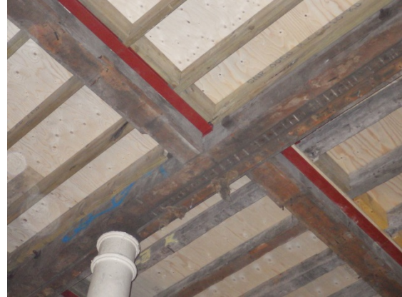
Plate 13 BL05 detail of floor structure above shows bolting visible for the east west beams
