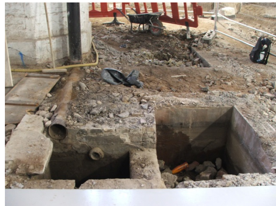
Plate 4 B.Z45 brick sumps
