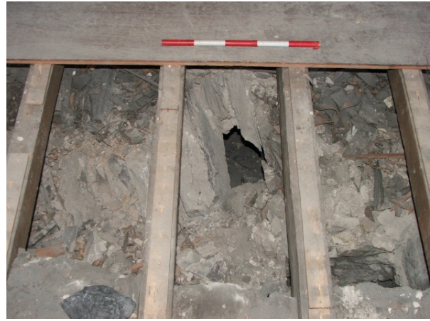
Plate 17 G.151 view of sub-floor vaulting showing small area of collapse allowing access for a camera
