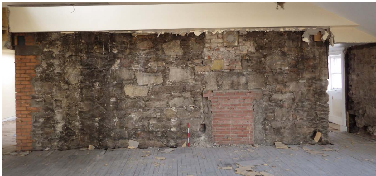
Plate 55 Room 2.363 west wall historic fabric with blocked fire/stove and stovepipe fixture above
