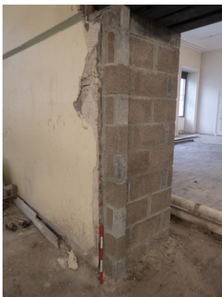
Plate 21 Room G.171/175 fireplace jamb cut by new door opening
