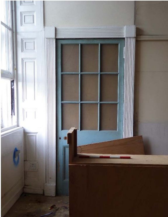
Plate 45 Room 1.298, southern wall showing exposed eastern relic door, leading to the “retiring room”
