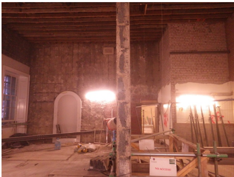
Plate 27 Rooms G.186-188 east wall with stove alcove and later brick partition walls
