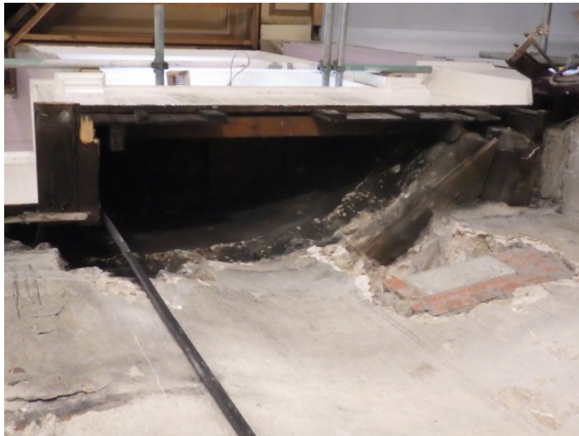
Plate 7 B.Z47 Evidence for circular stair well at wall head, view from below
