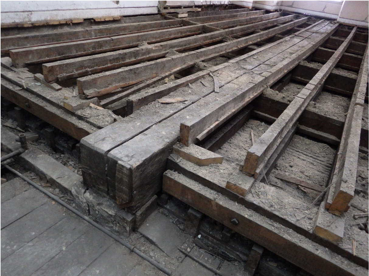
Plate 56 Room 2.365-8 floor structure shows main composite beam supporting floor structure and plaster ceiling below, note vertical lath and plaster of room below along edge of floor
