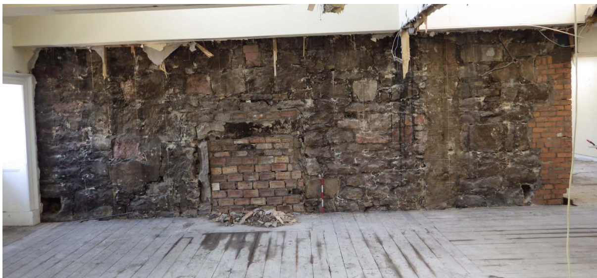
Plate 52 Rooms 2.358-9 east wall with blocked fireplace and brown rendered cut-back cross-wall to right.
