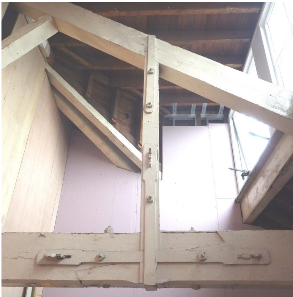
Plate 59 Roof structure 2.357-2.368 showing tie beam jointing with supporting strapping held with gibbs and cotters
