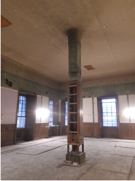
Plate 29 Room G.194, partitions removed, with column and early decorative scheme above modern ceiling line
