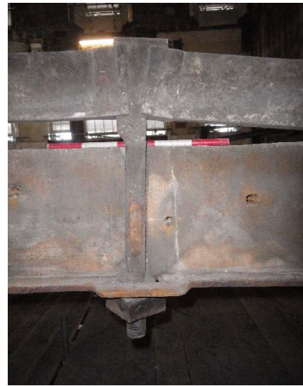
Plate 36 Room 1.288 detail of metal truss joint exposed
