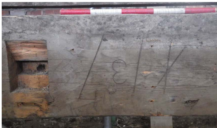
Plate 38 Room 1.288 main truss shows lesser joist mortise with bolt hole and race marks
