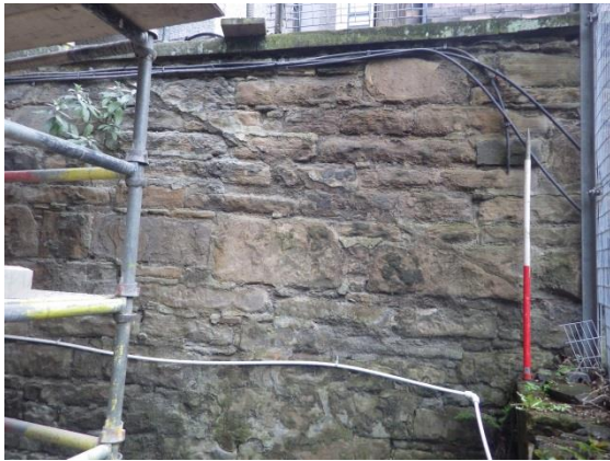
Plate 9 Rear yard, west boundary wall. Lean-to roof scar.
