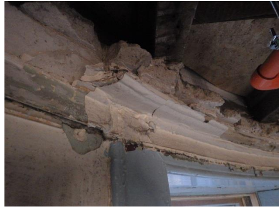
Plate 14 Basement, Room B.1, detail of corncicing above windows.
