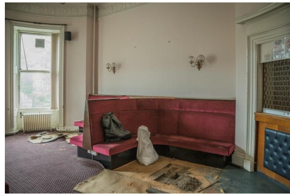
Plate 59 Room G.2, late Phase 4 fittings. Cooper Cromar.
