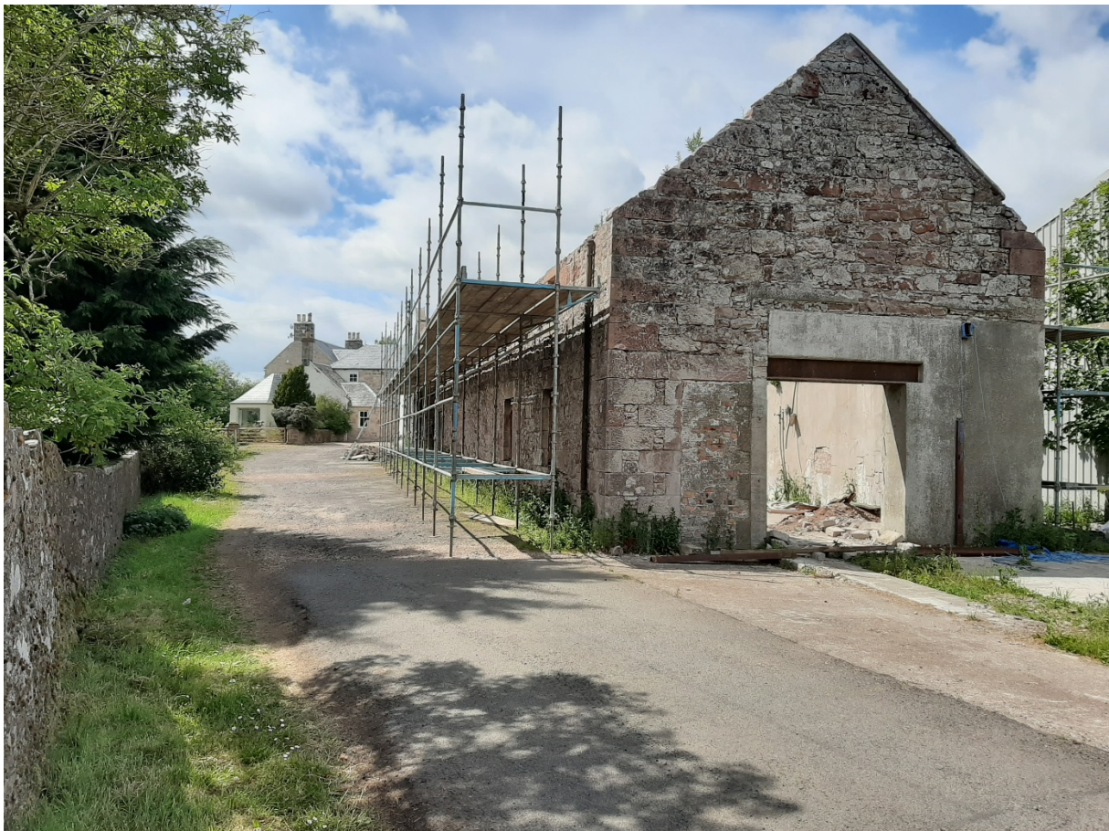
View looking westwards along the access road along the south side of the south range; farmhouse beyond
