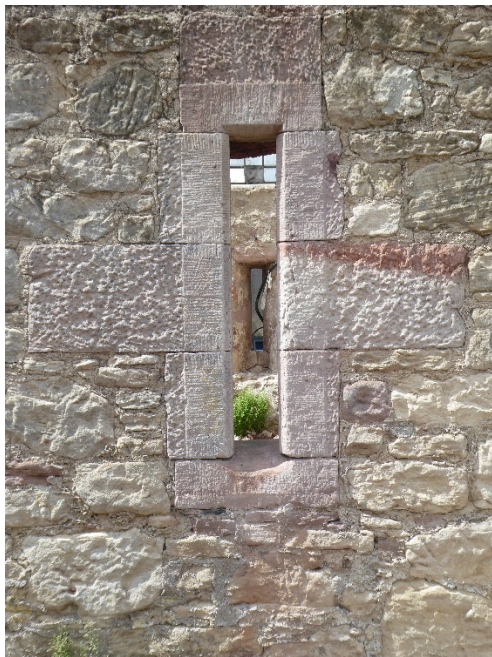
Plate 11 Narrow vent opening
