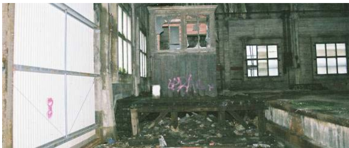
Plate 67: Secondary wooden platform and booth at NE corner of warehouse, upper floor, looking E
