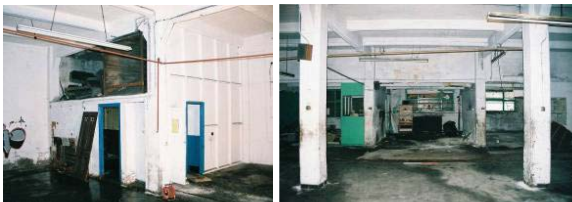
Plate 71: Secondary partitions in the NE corner of the lower ground floor of the warehouse Plate 72: Secondary partitions along the S elevation of the lower ground floor of the warehouse
