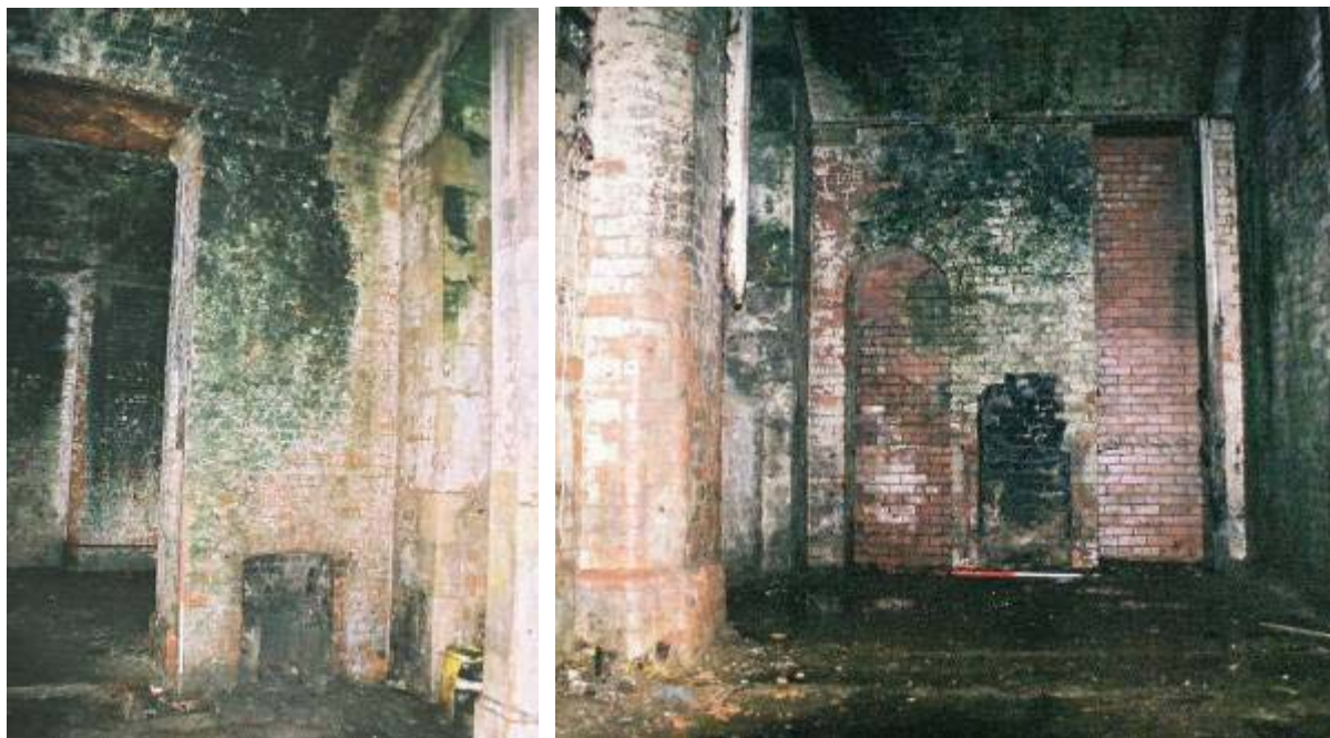
Plate 7: Fireplace in former office area, in 'aisle 2' of the Goods Station undercroft
