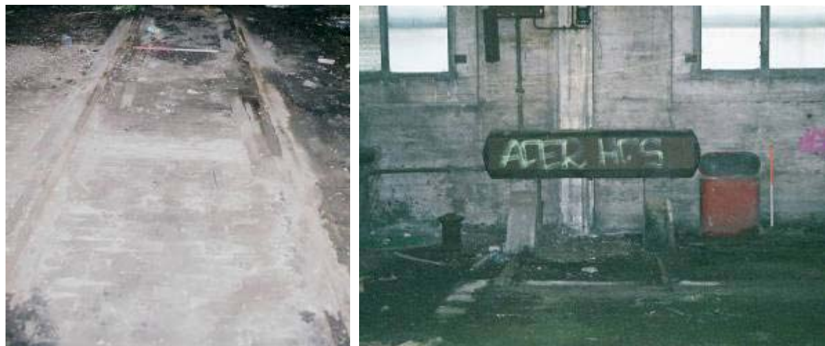
Plate 63: detail of track with wooden runners, in upper floor of warehouse, southern track Plate 64: detail of buffer at W end of N track in upper floor of warehouse
