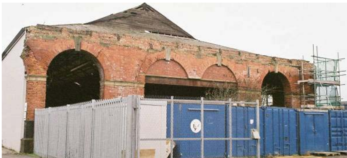
Plate 56: W elevation of Goods Warehouse, showing truncated arches of demolished Goods Station and modified central arches
