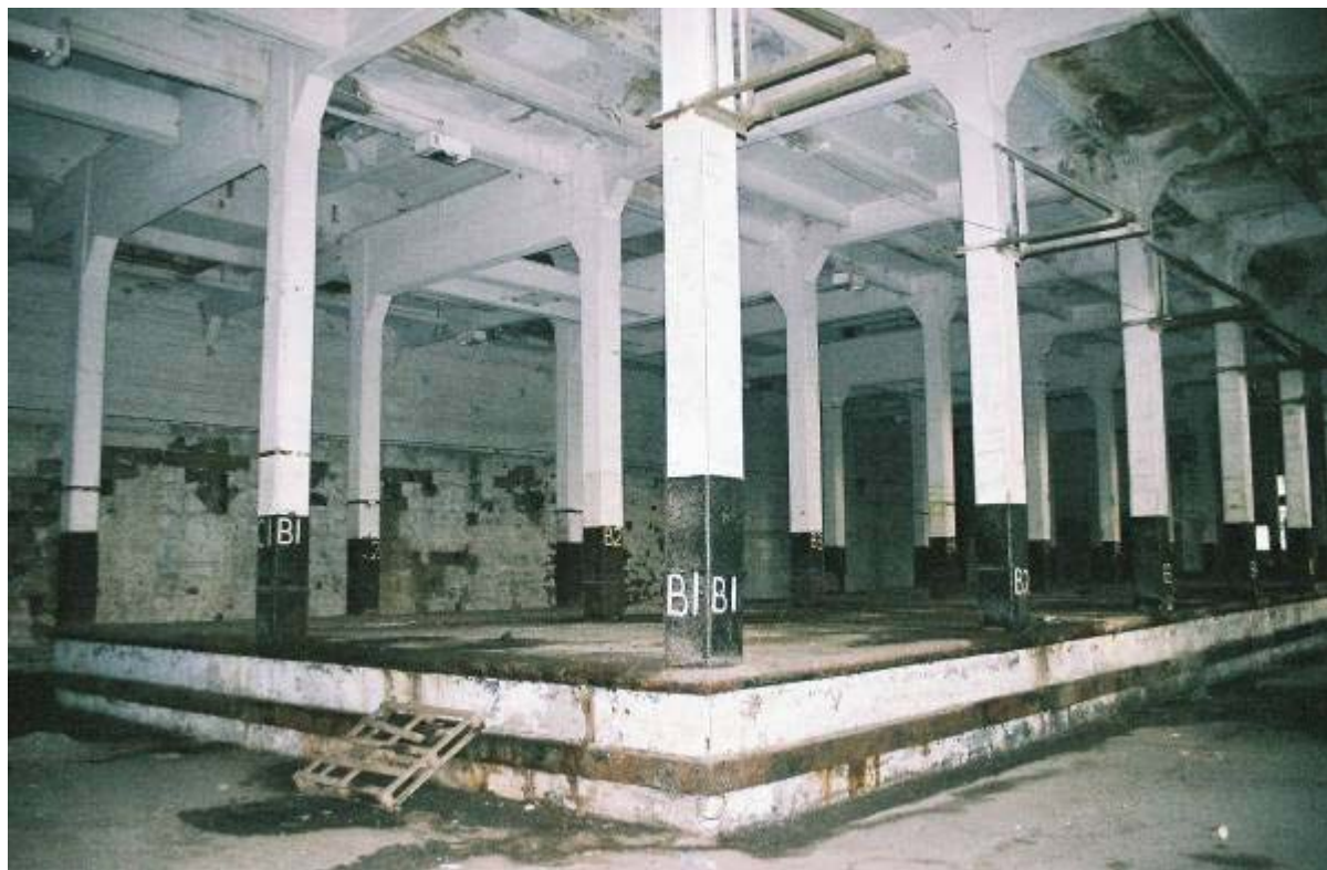
Plate 59: Goods Warehouse, ground floor platform with numbering system, also showing brackets and pulleys at the top of the piers
