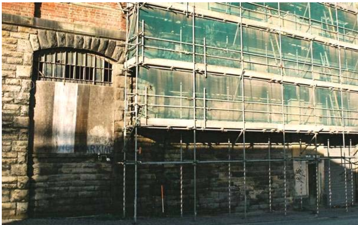
Plate 3: Sandstone infill between Goods Station and Goods Warehouse, lower floor facing onto Pottery Lane
