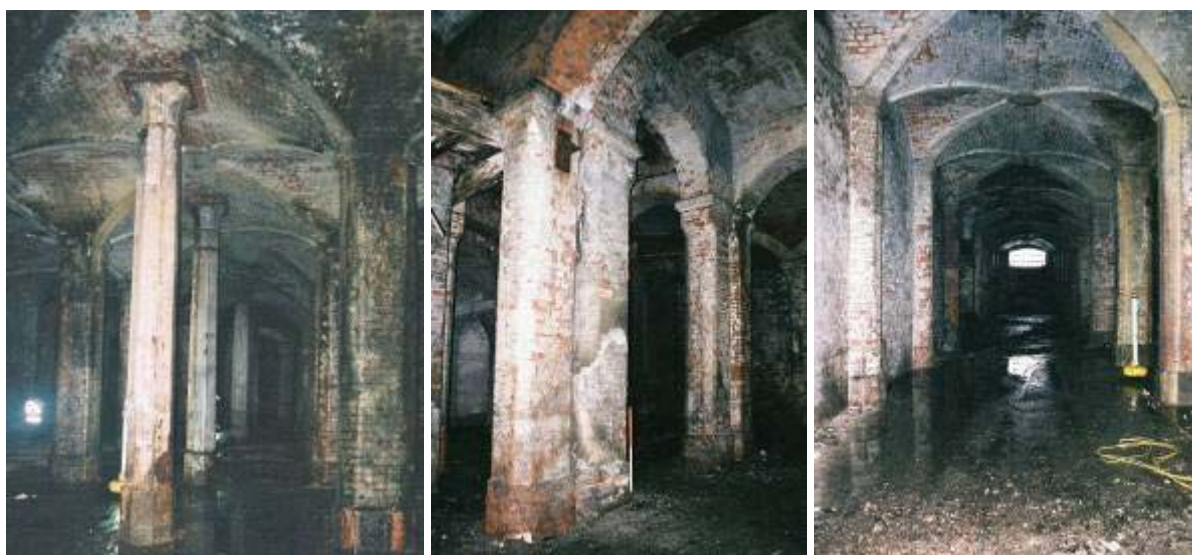
Plate 4: View of octagonal iron columns and brick piers in the Goods Station undercroft (looking N)
