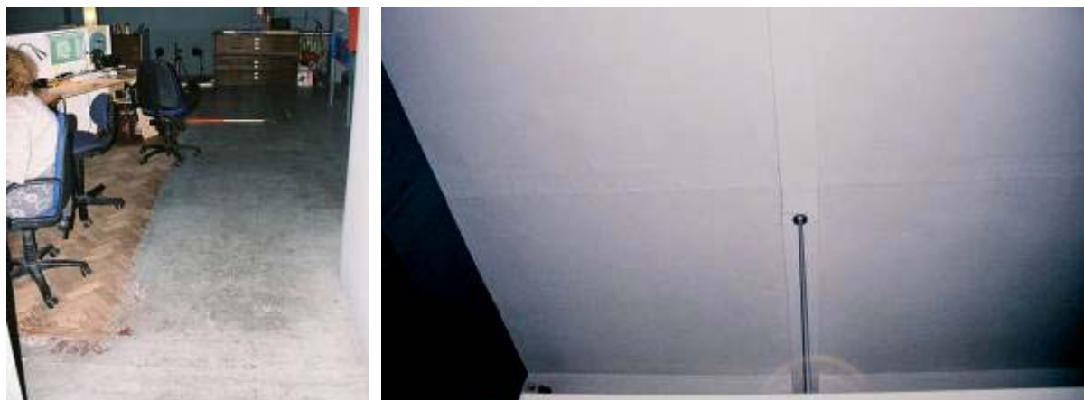
Plate 38: E-W orientated floor scar, indication former counter location in room 3 (separating the Carter's lobby from the Foreman's area)
