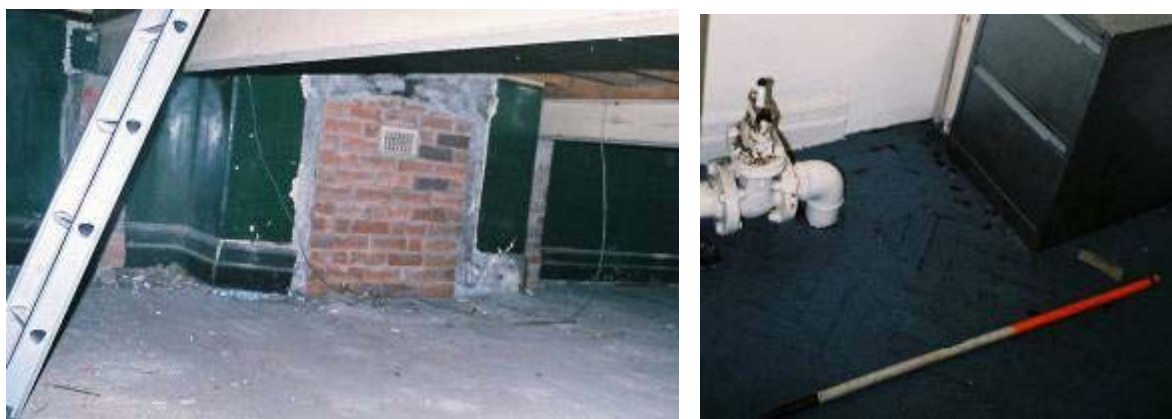
Plate 30: Bricked - in fireplace in Engineers waiting room (basement room B5/lower ground floor room 5)
