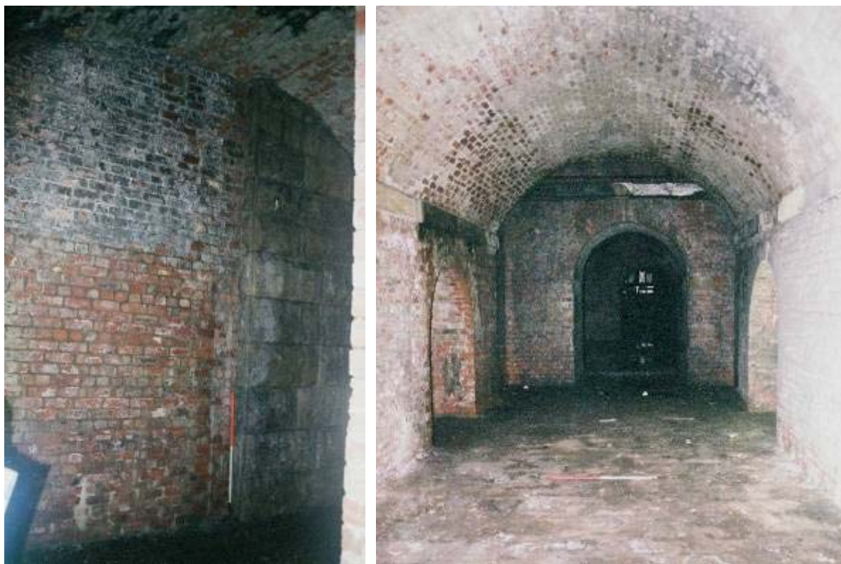
Plate 17: brick infilled arched opening, where the 1905 viaduct truncates southern façade Plate 18: secondary barrel vaulted chamber – substructure of 1905 viaduct
