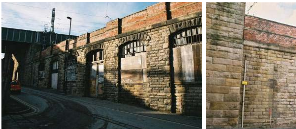
Plate 1: Southern façade, eastern end, of Forth Banks Goods Station Plate 2: Southern façade of Forth Banks Goods Station, showing blocked doorway where the façade is truncated by the 1905 King Edward Viaduct
