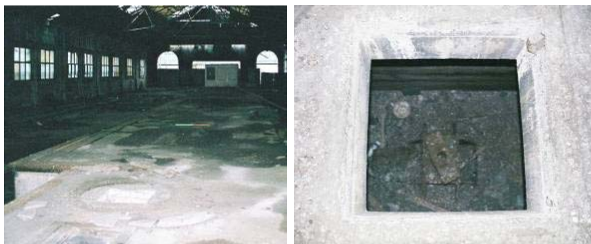
Plate 65: View looking W along the platform; the circular crane bases and boarded over hatches are visible Plate 66: View down open crane base, with footing for crane shaft at the bottom
