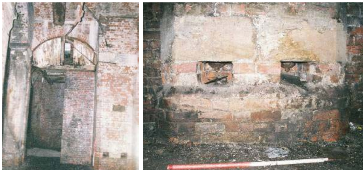
Plate 15: Gas pipe with fitting for gas lamp, extending around the ceiling of the Goods Station undercroft Plate 16: Detail of brick pier, with fittings at base, for controlling the lighting system?
