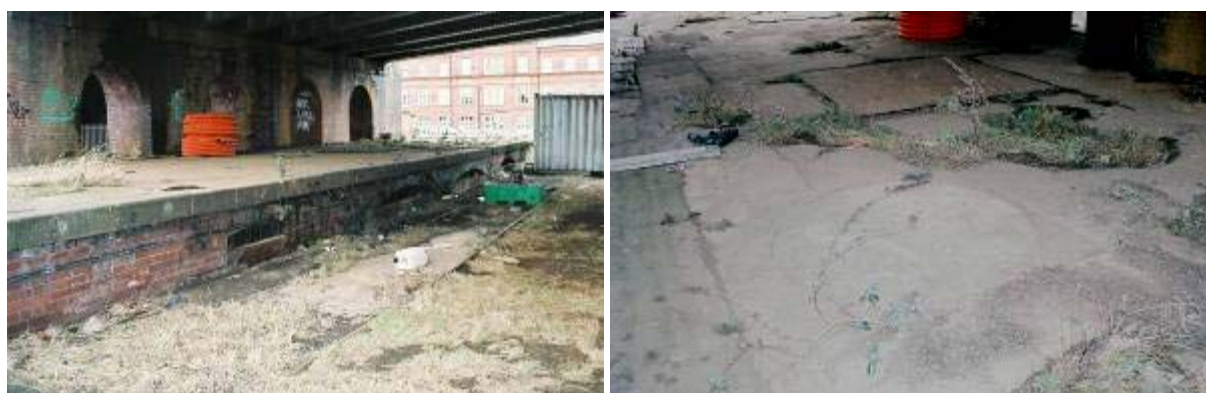
Plate 11: View of remains of platform and rail tracks in the car park area, located above the Goods Station undercroft; these would have originally run through the Goods Station.
