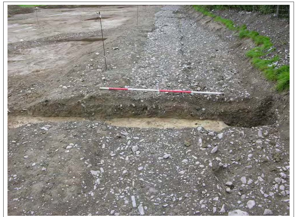
Plate 28: View of Section two excavated through road surface onto natural clay. Looking SE. Scale 1x2m
