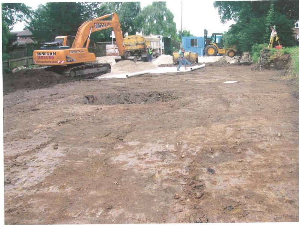
Plate 1: Surface stripped, with the machine on spoil, terram being laid and stone being delivered. The disturbed area just above centre is the void left by the garden pond. Looking west towards Duffield Road.
