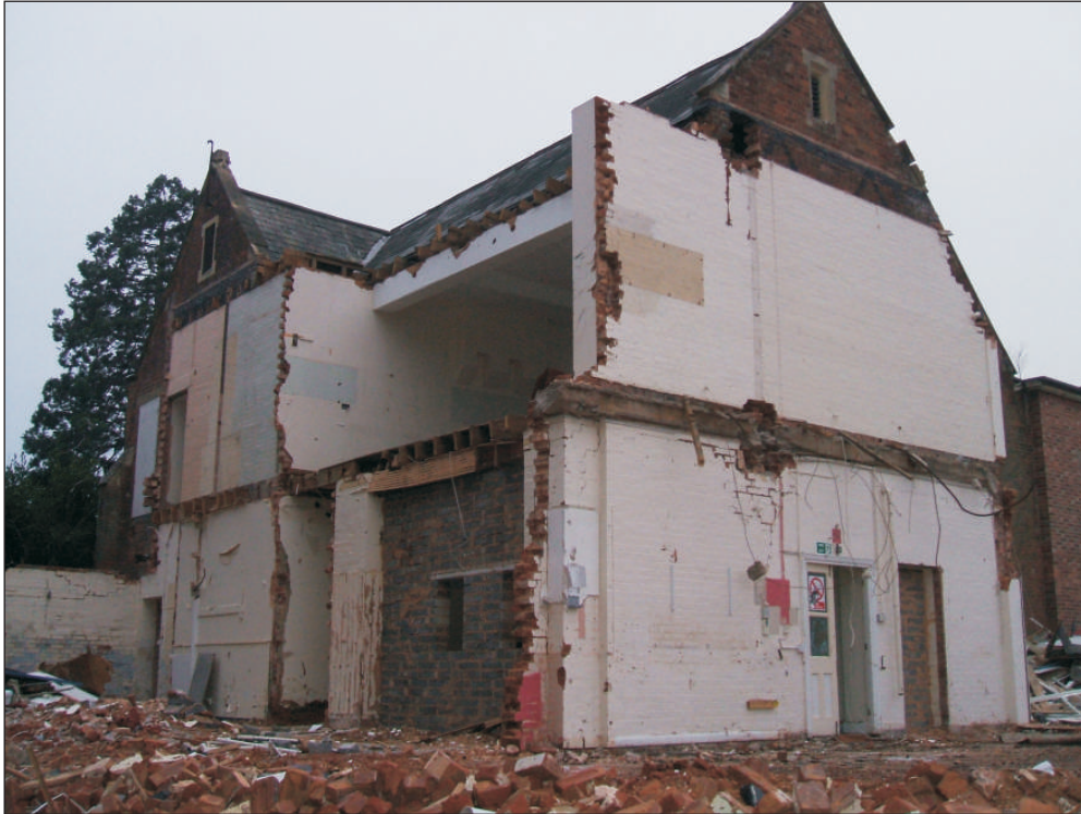
Plate 1: The Episcopal School during demolition of the south 1936-8 wing, showing exposed now-blocked original window in the south elevation, viewed from the northeast.
