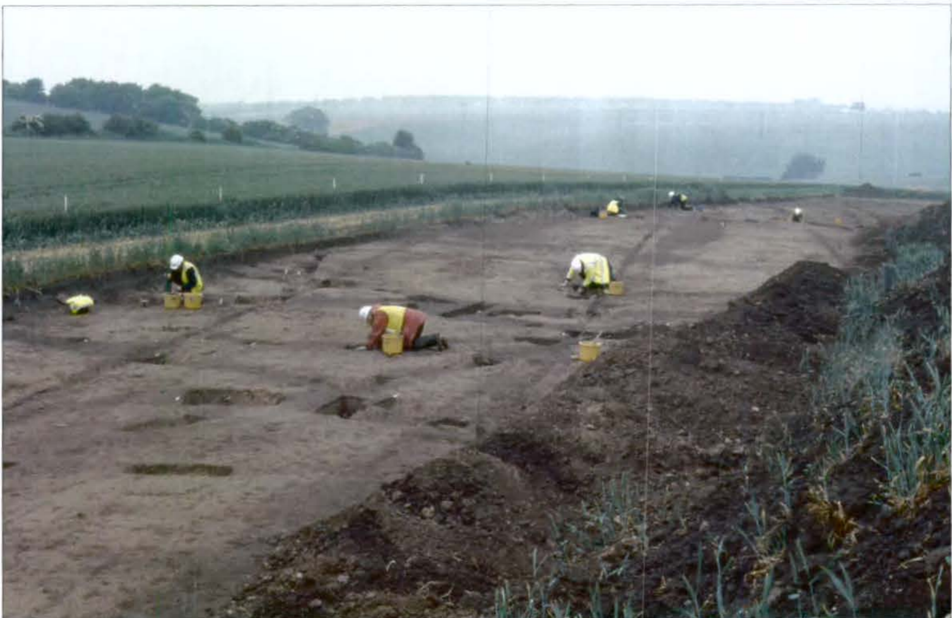
Plate 2 Cowpen Bewley to Warden Law pipeline: Pig Hill, excavation of archaeological features by hand.
