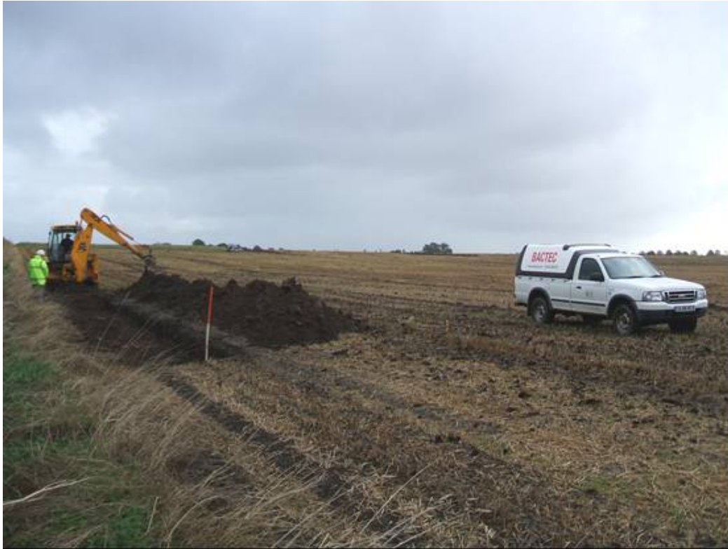
Plate 1 Overall view of trench under excavation, being monitored for live World War 2 ordnance
