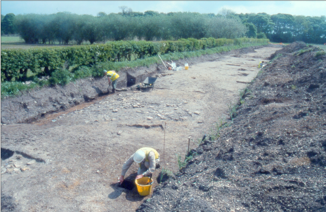
Plate 1: General view of the Low Common Lane excavations looking south-east along the pipeline corridor
