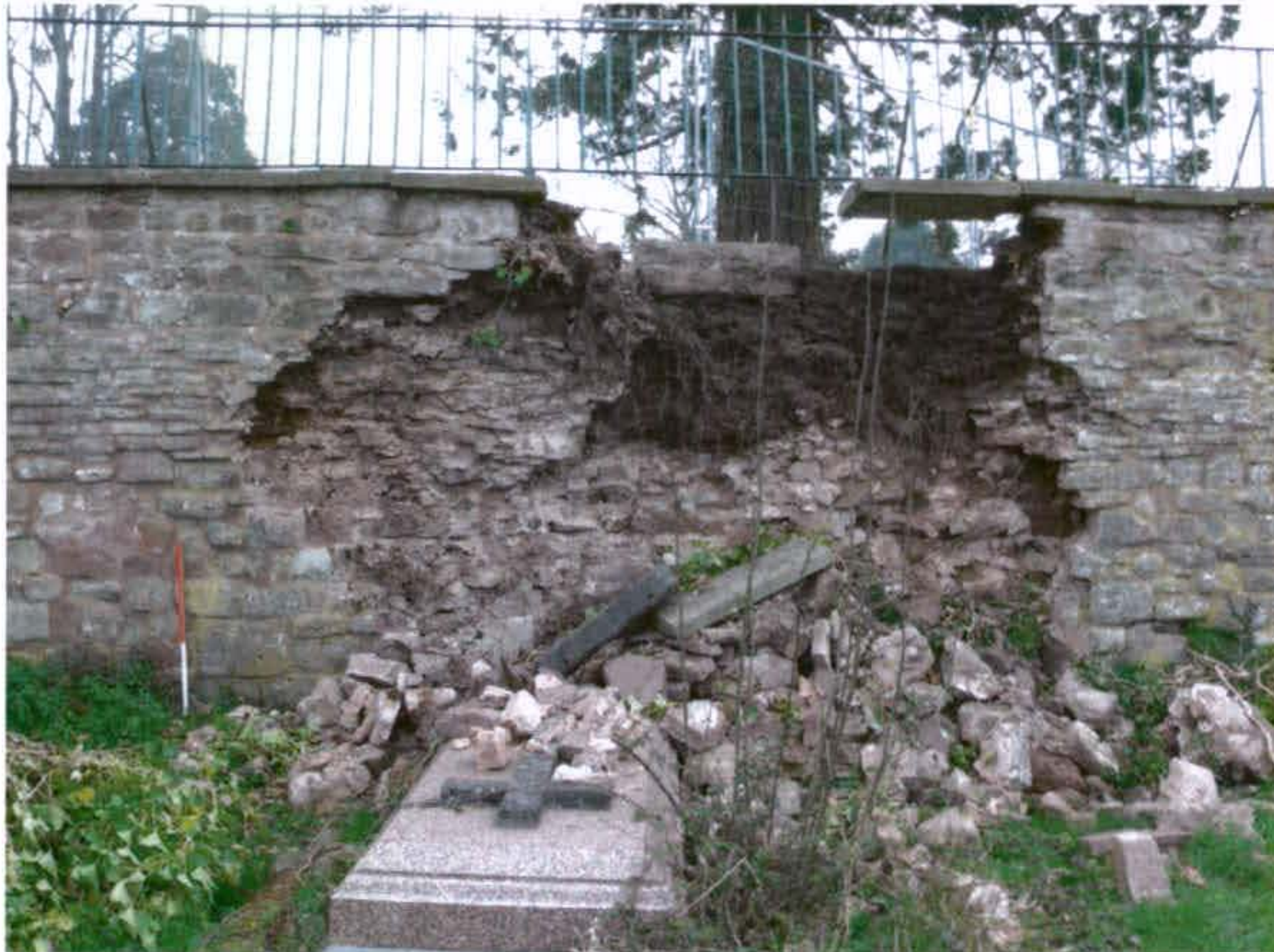
Plate 1: Picture of collapse along the Prospect boundary wall
