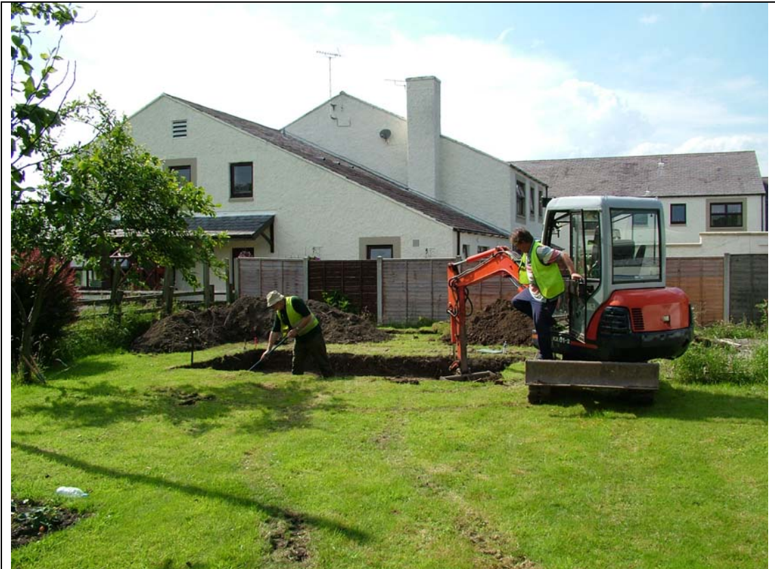
Plate 1. Trenching area, north-west corner of site with view of Dutton Brook House.
