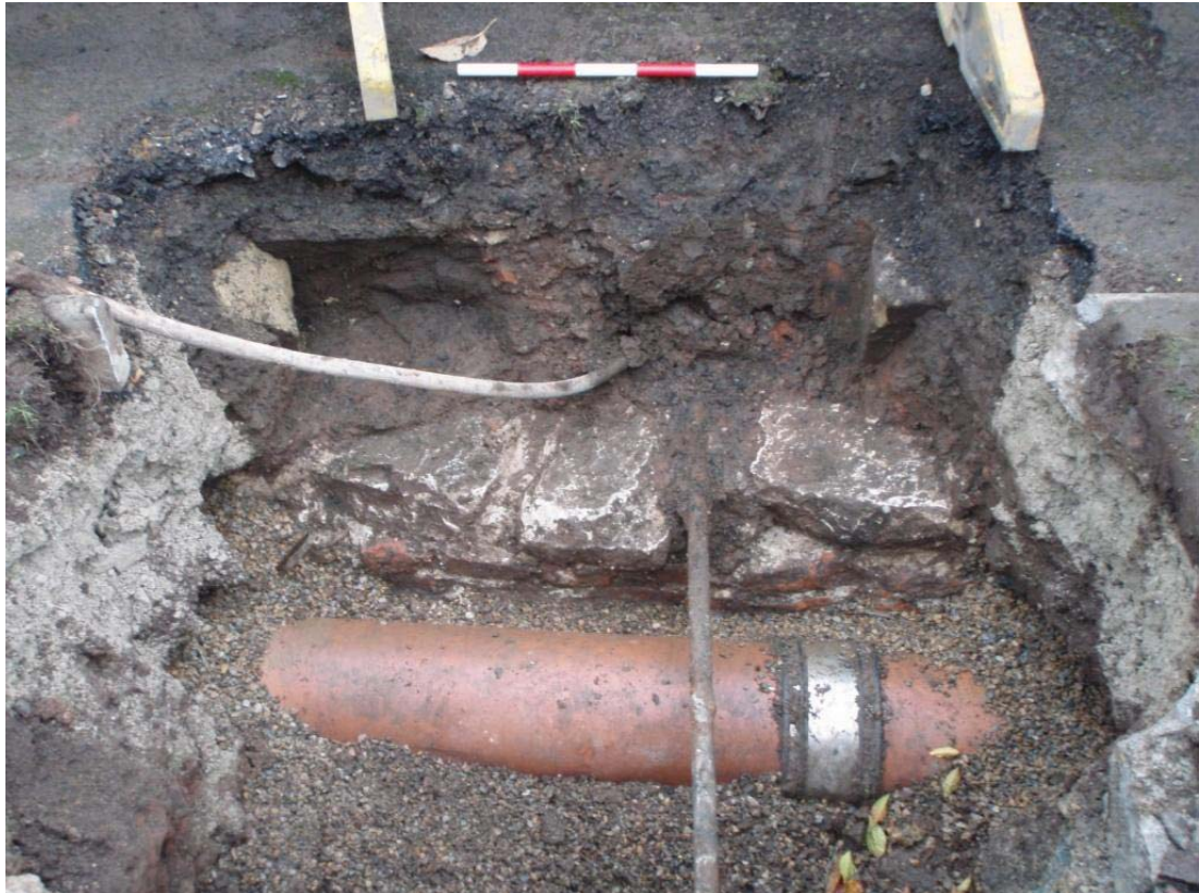
Plate 8 Stone and brick structural remains in Trench 37, looking SW. Note that the stubs of later kerbing slabs can be seen towards the upper parts of the sections to the side of the trench (removed between these points).
