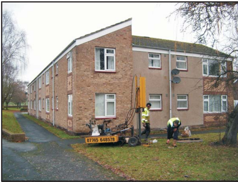
Illus. 15: The location of Borehole 4 at the south-east corner of Trinity Court, viewed from the east side.
