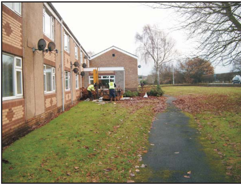
Illus. 12: The location of Borehole 3 on the south side of Trinity Court, viewed from the west.
