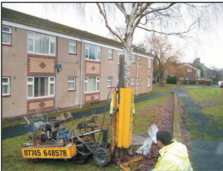
Illus. 18: The location of Borehole 5 on the south side of Trinity Court, viewed from the south-west.
