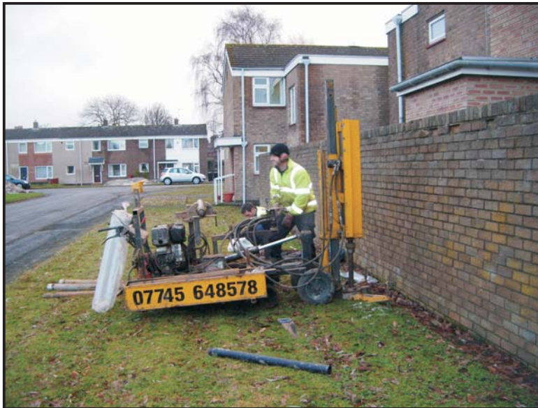
Illus. 07: The location of Borehole 1 on the north side of Trinity Court, viewed from the west.
