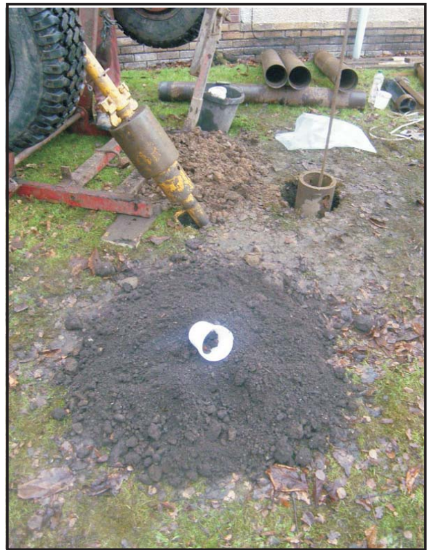
Illus. 29: Borehole 7 spoil-heap from the initial hand-dug test pit, from which fragments of Roman pottery and brick were retrieved.
