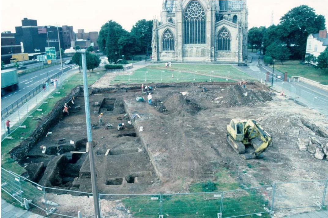
Plate 1. General view of the Church Walk excavation, looking west towards St George's Minster, before the Site was extended to the north.
